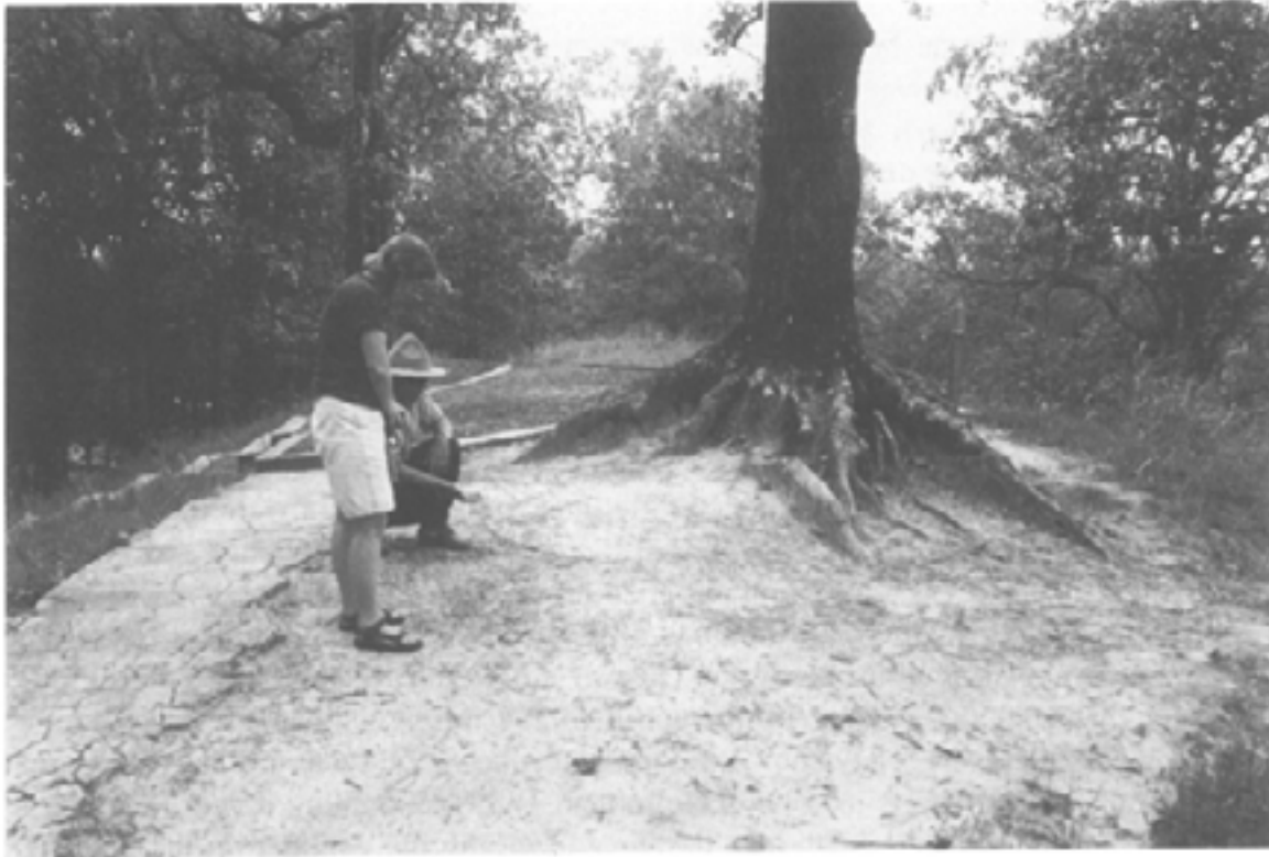
Figure 32 Crest of the bird-effigy mound, Poverty Point, showing unsatisfactory cemented path on left, and foot-erosion of summit. The extent of erosion is indicated by the exposure of the roots of the tree centre.
