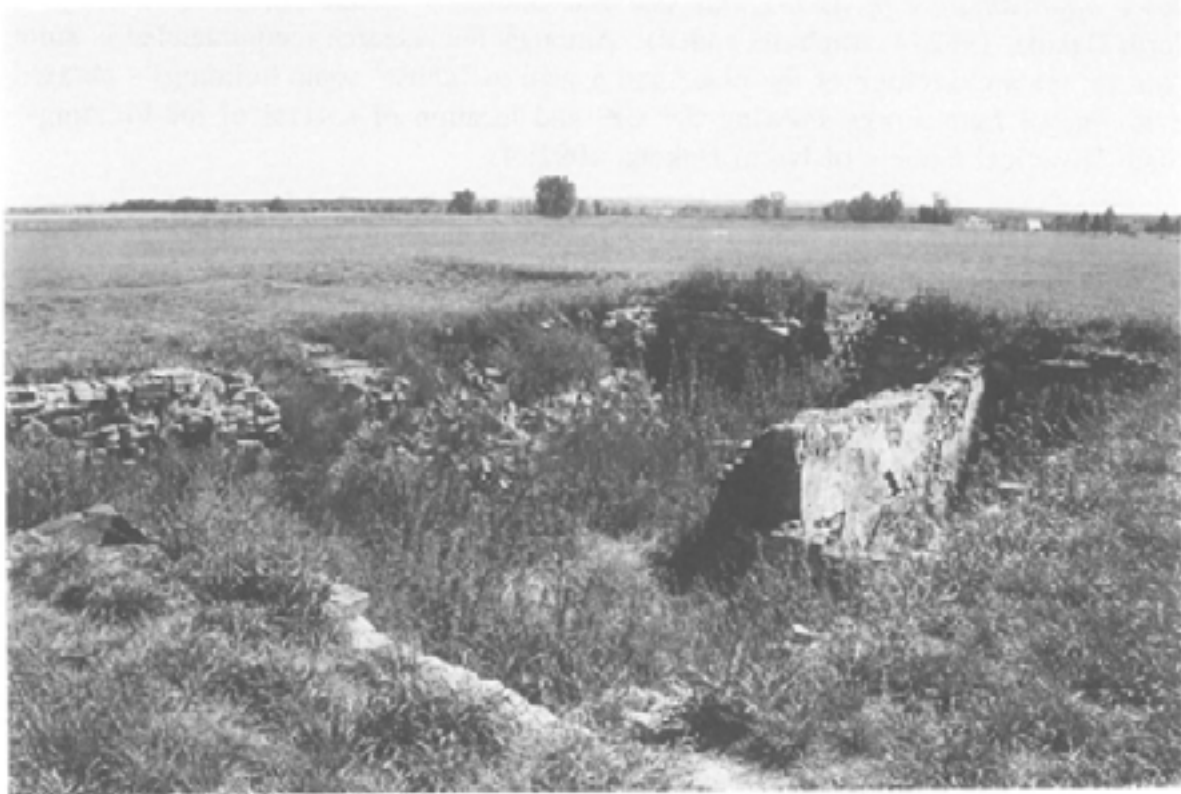
Figure 13 Cellar of the officers' quarters, Fort Buford. The foundations of the building, at left, are being mowed over and damage is accumulating.
