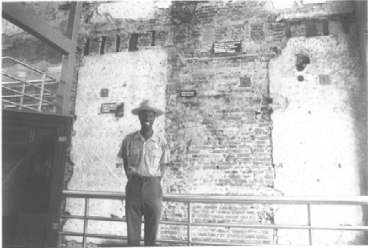
Figure 36 Exposed wall in the late 18th century "Market Street" or "Moyety" houses. This wall is exposed in one skeletal unit of three units reconstructed on the site. Exposed on this wall is the original plaster finish, the demolished chimney, and the joists of a floor (at top). At left are modern steel joists supporting a stairwell to allow a view of the full 3-storeys of the original wall.
