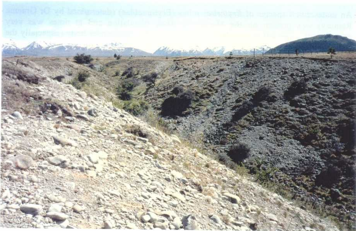
Figure 9 Tekapo Canal, high terrace lateral gully showing degrading embankments of fluvioglacial deposits.
