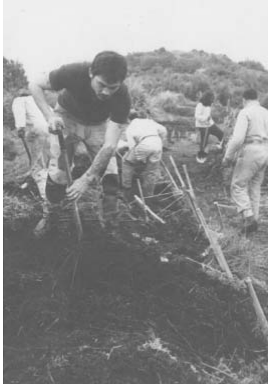
Figure 7 Filling behind the formwork of stakes and manuka brush on the eastern perimeter of the site.
