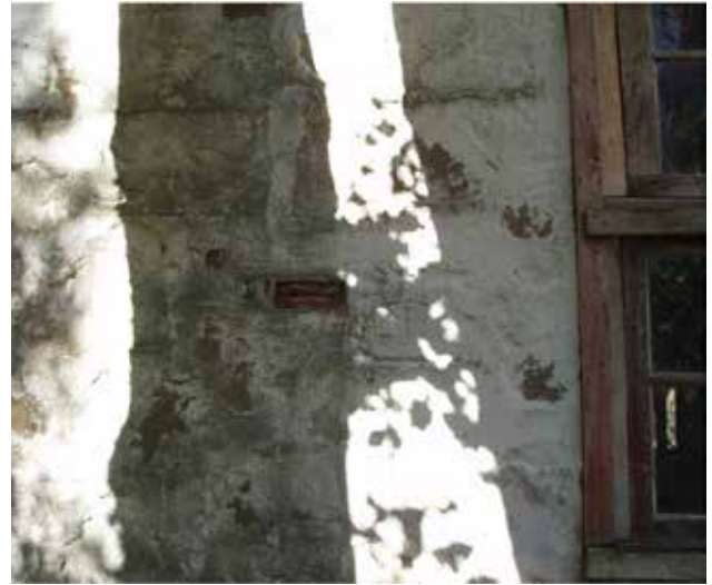
Figure 45. One of the beams set into the exterior west wall of the White Hut. Photo: Katharine Watson.
