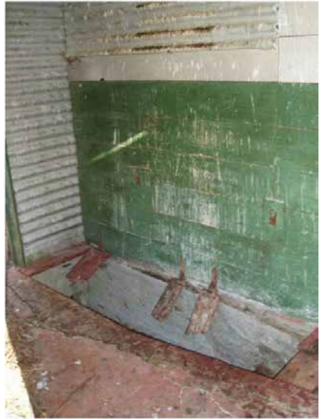
Figure 32. The location of the fire that fed the central heating in Room 3 of the Barkers' house. Photo: Katharine Watson.
