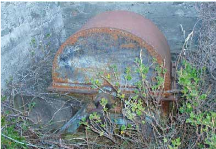
Figure 64. The Pelton wheel and its cover in the power house. Photo: Katharine Watson.
