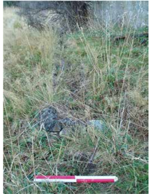
Figure 63. The concrete-lined drain that collected excess water from the power house. Photo: Katharine Watson.
