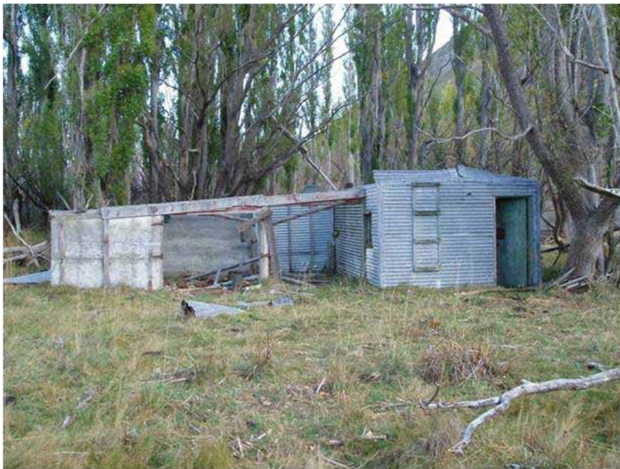
Figure 26. The east elevation of Phase 1 of the Barkers' house, showing the shallow pitch of the roof and the ladder for roof access. The concrete section to the left is Phase 3 of the house. Photo: Katharine Watson.
