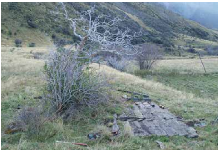
Figure 55. The collapsed remains of the hockey rink shelter on the bank above the hockey rink, looking northeast. Photo: Katharine Watson.
