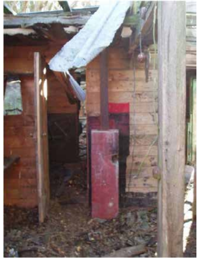
Figure 29. A flue associated with the central heating in Room 1 of the Barkers' house. Photo: Katharine Watson.
