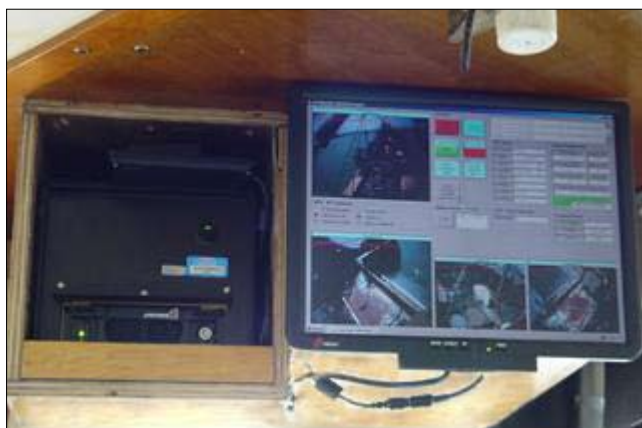
Figure A1.1. EM control box and user interface installation on V1 (ceiling mounted).
