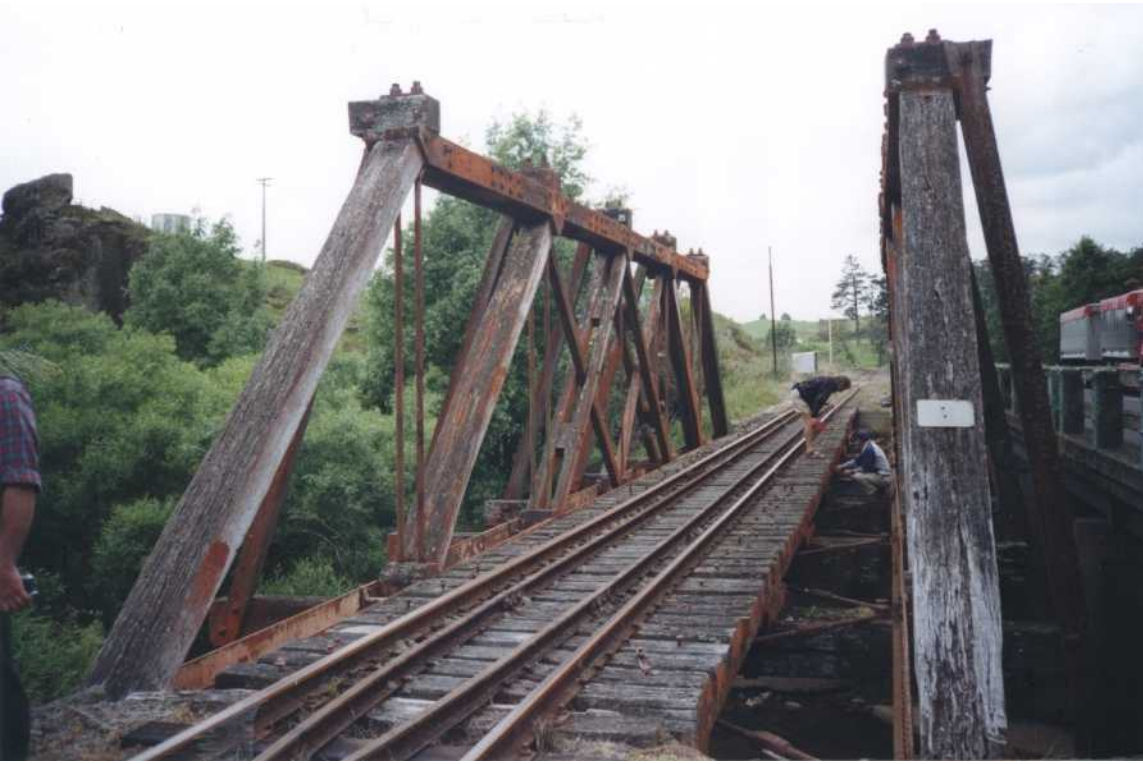
Figure 4. General view of the bridge from the Waikino end, before water-blasting and treatment started. There was extensive orange algae and lichen on many of the components as well as deep fissures and occasional deeper decay.
