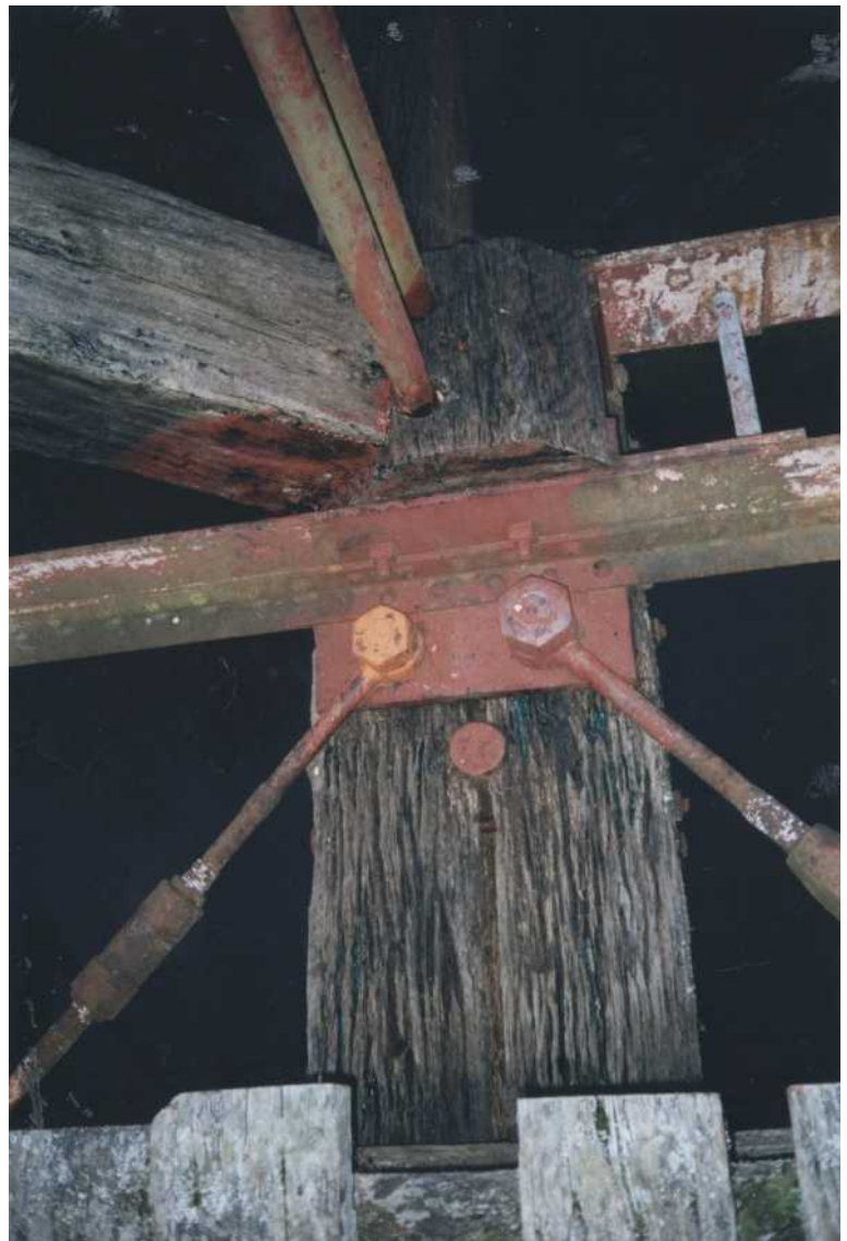
Figure 7. The upper surface of transom 17, compression block 37 and the lower end of queen strut 3, six days after application of CN Emulsion. The surface has almost returned to its original grey colour; there is some darkening and traces of CN Emulsion in the fissures.
