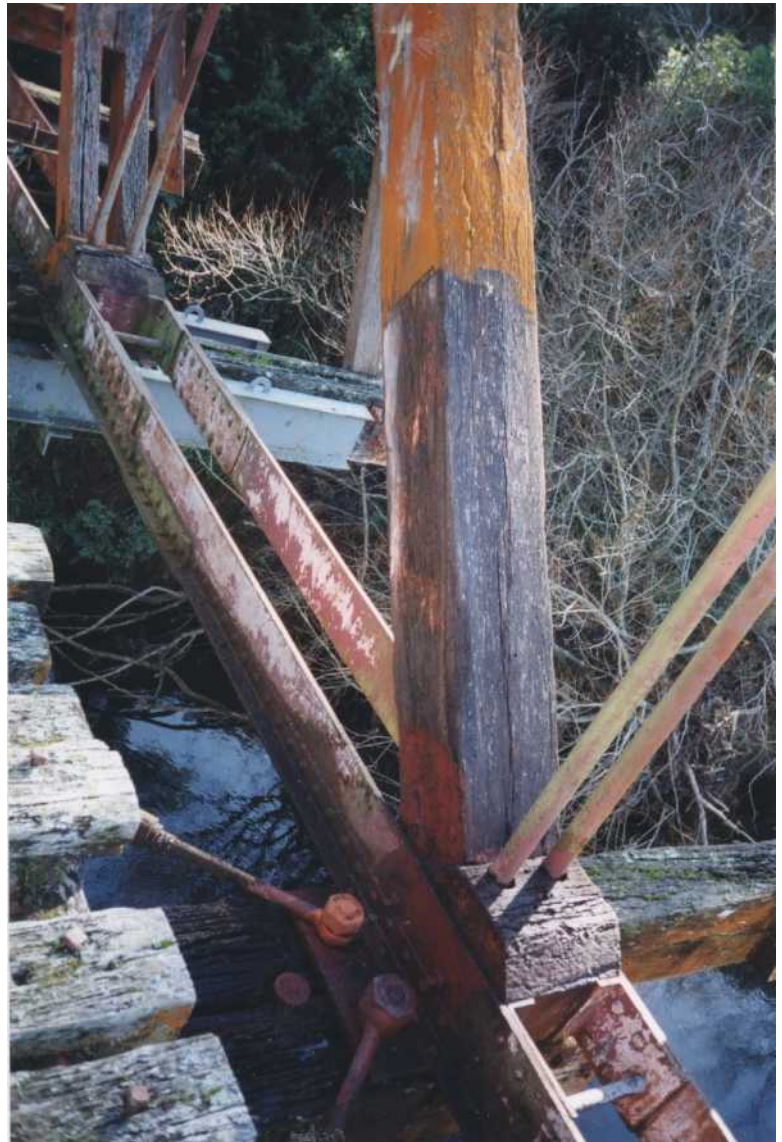
Figure 5. Initial water-blasting test on queen strut 3 and compression block 37. Water-blasting removed the orange algae, lichen, debris and most of the moss and vegetation growing in fissures in the beams. The original red primer on both the metal and wooden components was not all removed.
