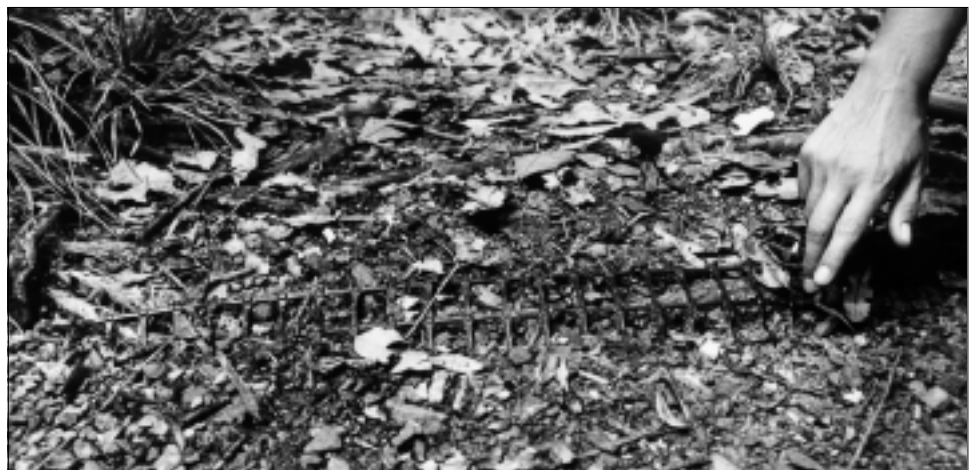
Figure 23. Open-pored moulded geogrid provides a base for well bedded angular gravel protecting a midden on this track in the Ōhope Scenic Reserve, Whakatāne.
