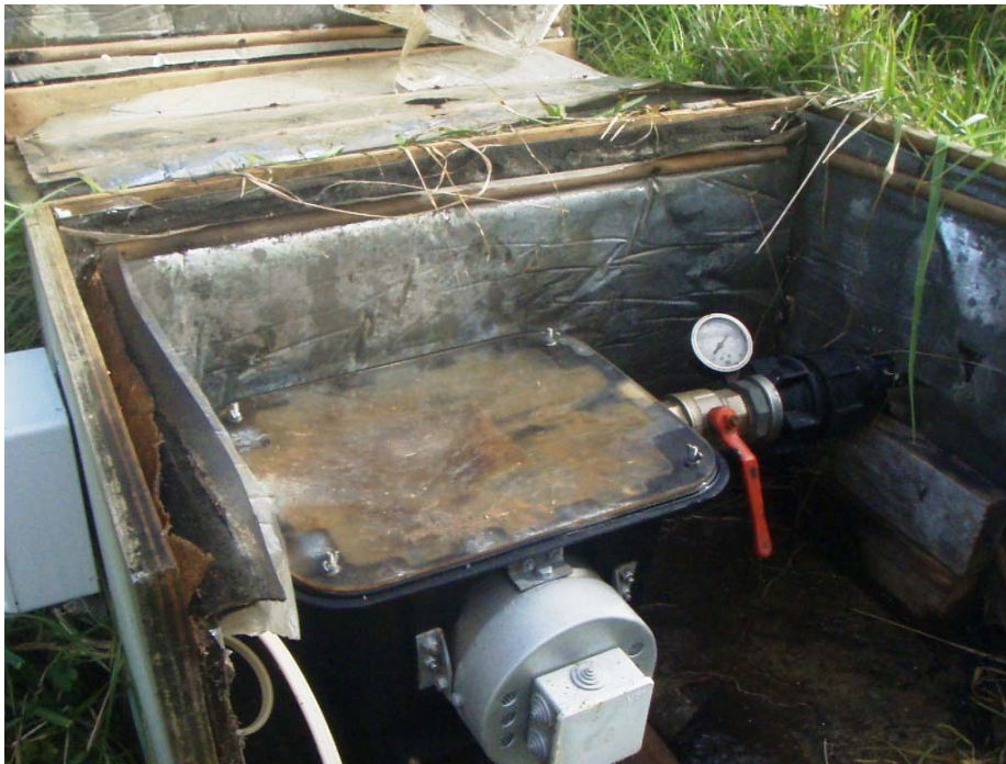
The Pelton wheel driven micro hydro electricity generator which supplies much of the power for Whatipu Lodge, run by the gravity fed water supply. Photo supplied by Raewyn Bennett.
