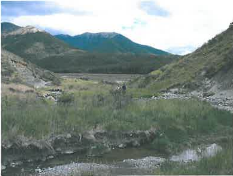
Figure 3: Eroded bank at stream in the gulley downstream of the terminal building.
