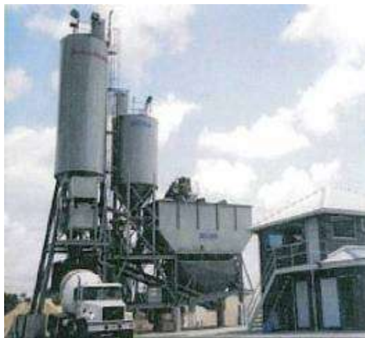
Figure 2: Example of concrete batching plant
