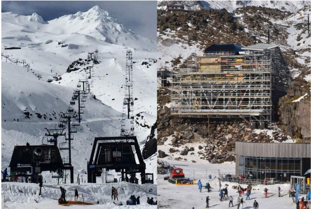
Image 4 Left – View of the Movenpick and Parklane fixed-grip chair drive stations currently at the base of Türoa. Right – View of the Whakapapa Gondola storage and drive station at the base of Whakapapa (under construction)
