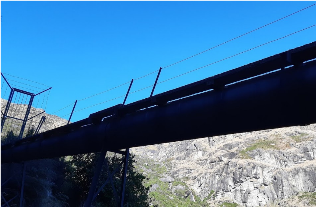
Figure 16. Pipeline structure for Wye Creek hydro-electric station. Photo: Carl Walrond, DOC.
