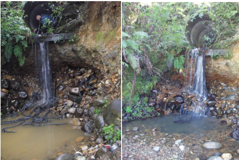
View from below the culvert during installation (left photo) and completed retrofit (right photo)
