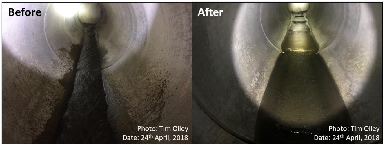
Figure 2. Lower section of the Reservoir Creek culvert before and after Flexi-baffle installation.
