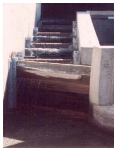
Figure 2. Pool/weir fish pass installed on the outlet of the Tekapo Canal. (April 1992; Source: Mark Webb)
