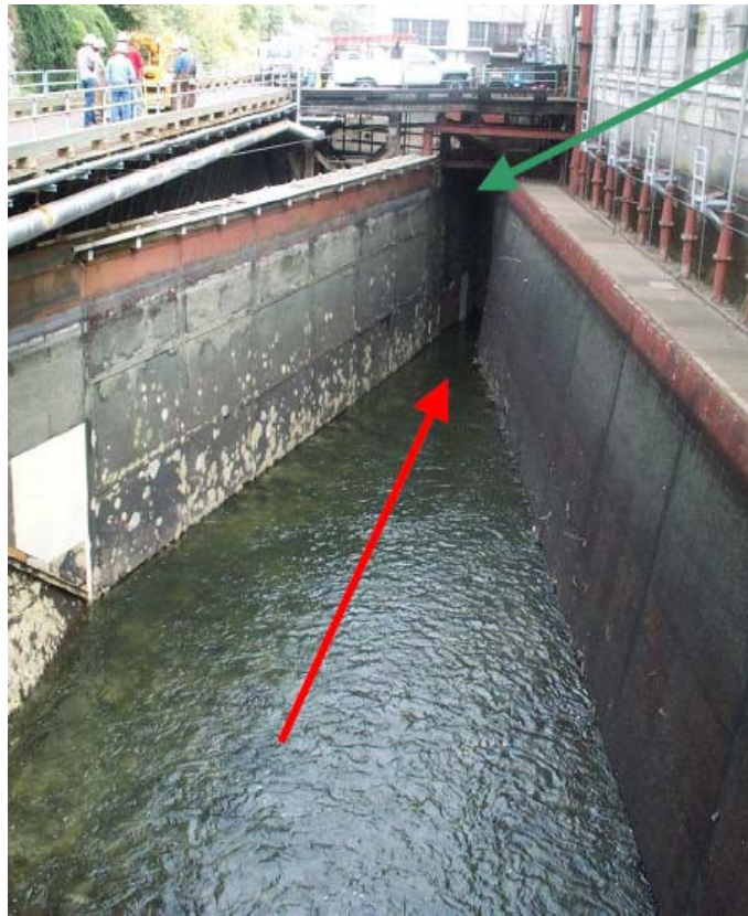
Figure 18: Flat screen barrier. Red Arrow points to Fish bypass entry at flat screen. Green arrow indicates height of slot to handle water level fluctuations (USA).
