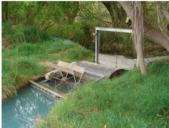
Figure 1: Drum screen, rotary intake.
