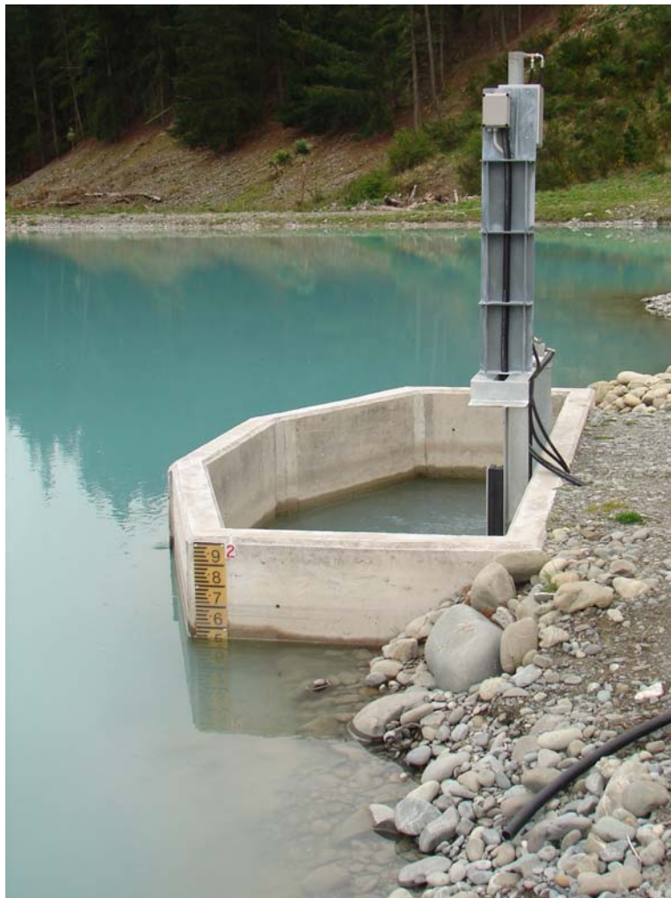
Figure 23: General view of gallery intake
