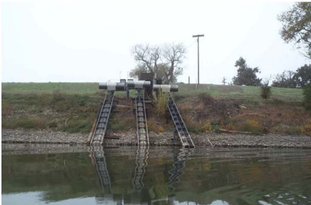
Figure 7: Raised cylindrical screens (California)
