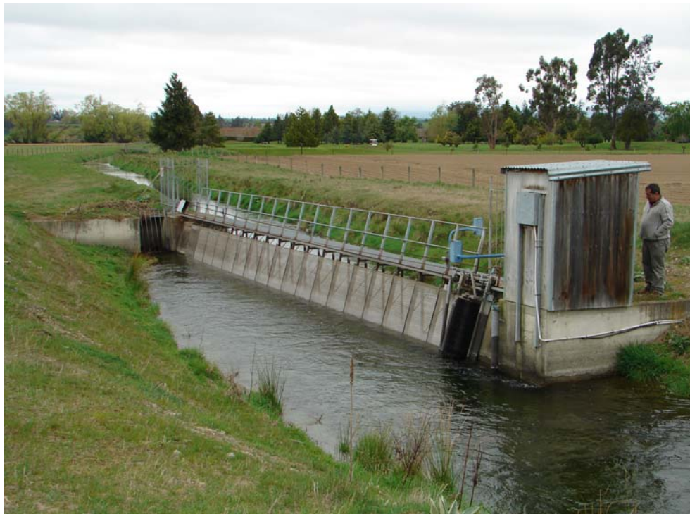
Figure 26: Flat screen intake (Levels Irrigation scheme)
