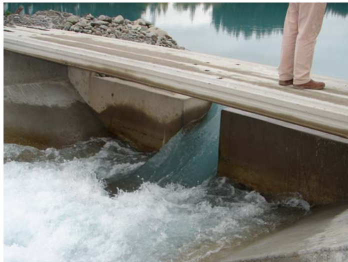
Figure 24: Bypass intake structure – “bell mouth” shape of the entrance ensures gradual increase in the by-pass flow while high flow plus high velocity in by-pass channel means no opportunity for fish to return to intake zone via this passage.
