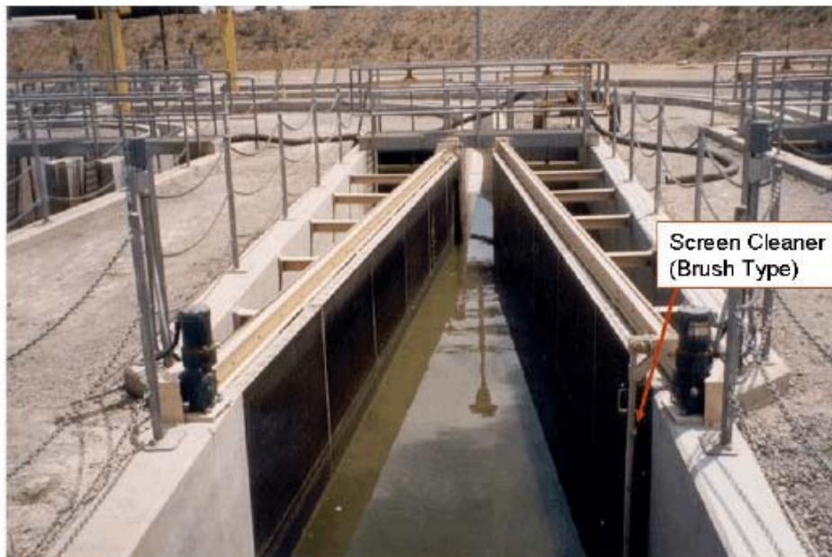
Figure 2: Example of flat plate screen “V” configuration, with a terminal fish bypass. – Abstracted water exits via side chambers behind screens while bypassed fish continue straight ahead and return to main channel.
