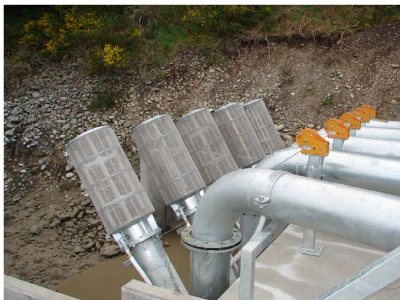
Figure 27: Self cleaning pump intakes
