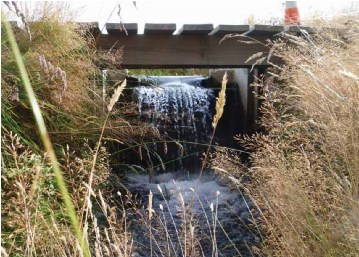
FIGURE 9 Built barrier installed at Fraser Spring, Twizel in the Waitaki catchment to prevent trout accessing bignose galaxias and lowland longjaw galaxias habitat.
