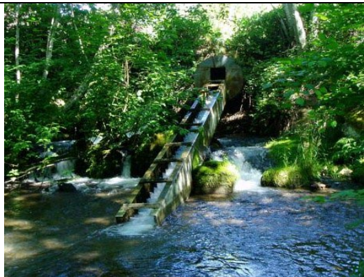
Figure 7.5. Photo examples of vertical slot fishways.
