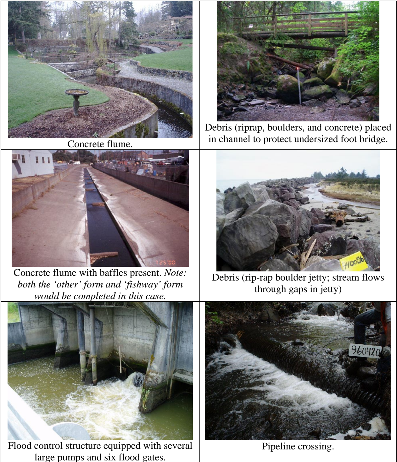
Figure 5.1. Examples of some previously inventoried miscellaneous obstructions.
