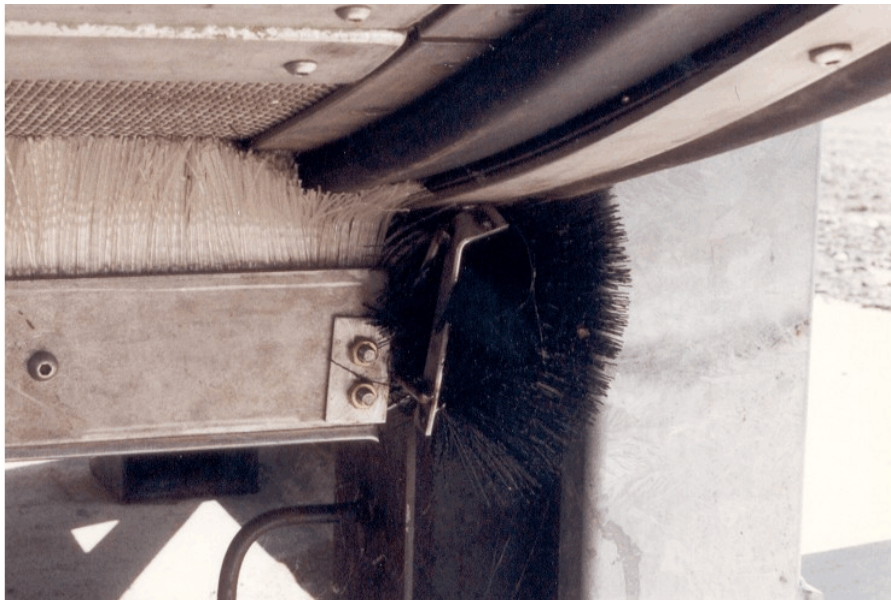
Figure 72.—Drum screen bottom brush seals and side neoprene seals.
