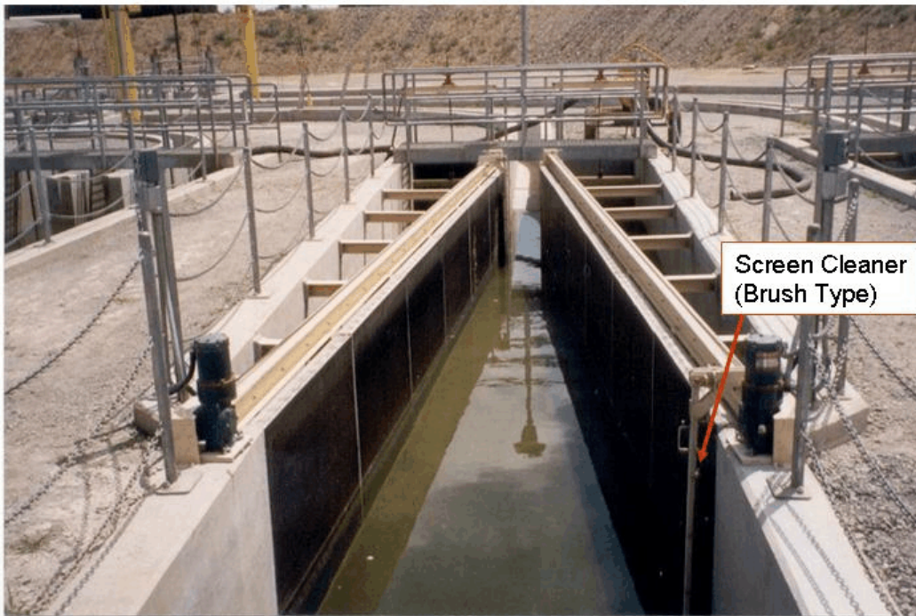
Figure 10.—Flat plate screen “V” configuration with terminal fish bypass – Red Bluff Fish Evaluation Facility, California.
