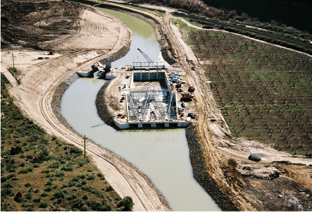
Figure 35.—Site isolation and dewatering for construction, Highline Canal Fish Screen Facilities at Grand Junction, Colorado.
