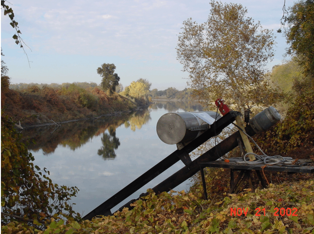
Figure 17.—Track mounted, retrievable rotating cylindrical screen with fixed brush cleaner (intake screens incorporated).
