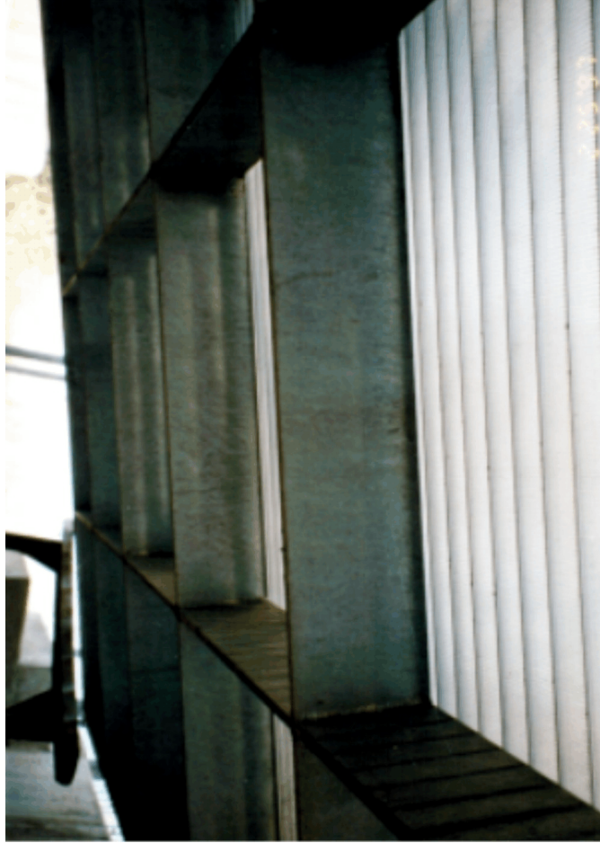
Figure 62.—Downstream view of flat plate screening panel, support frame, and screen.
