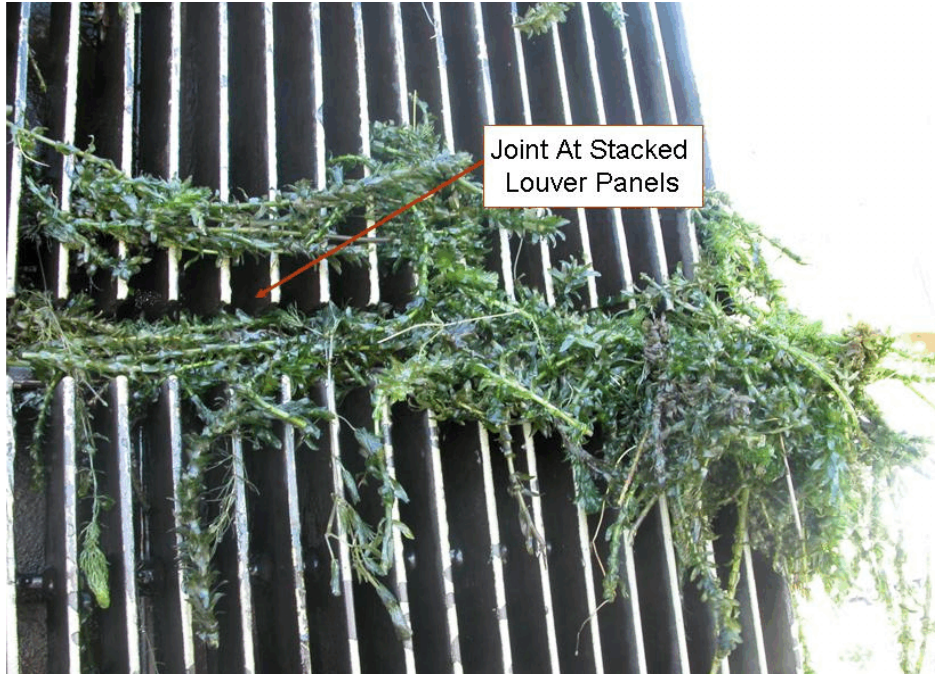
Figure 95.—Fouling of Tracy Fish Collection louvers by Egria.
