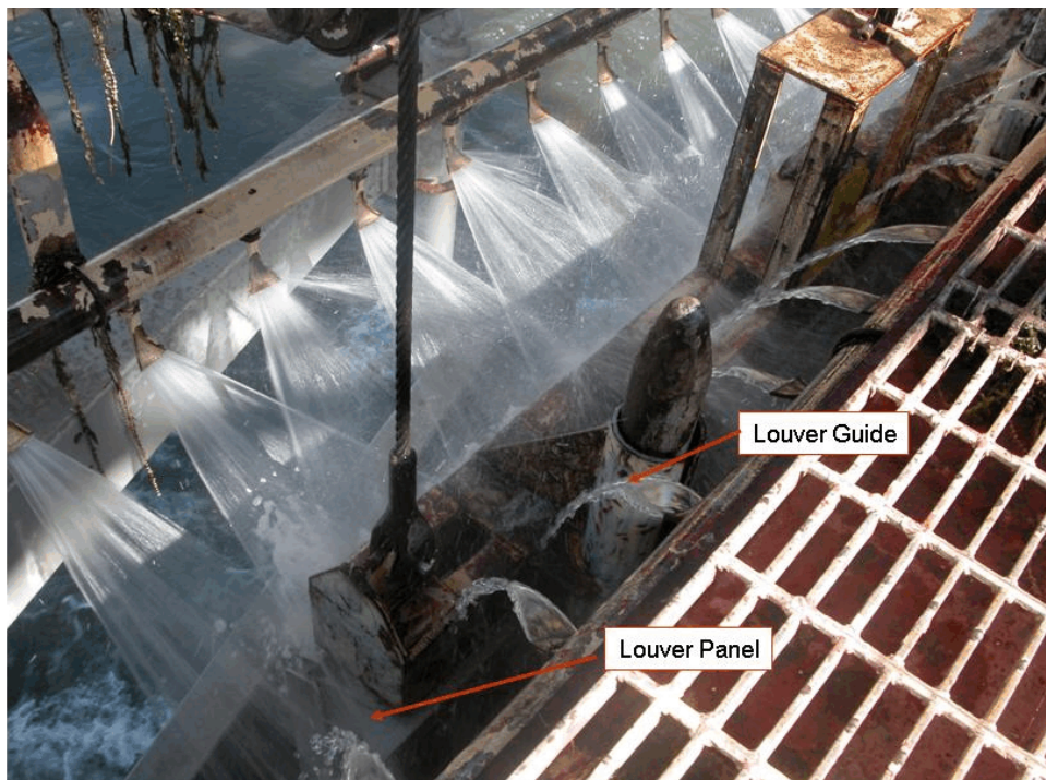
Figure 96.—Spray bar used to clean louvers at Tracy Fish Collection Louvers (downstream spray bar not operating).
