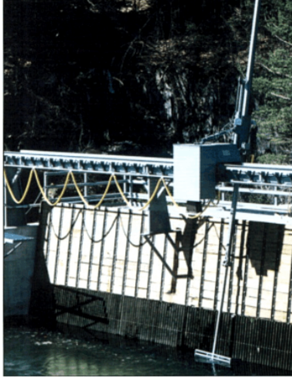
Figure 58.—Mechanical driven rake on trashrack structure (Atlas Polar – Hercules Hydro Rake).
