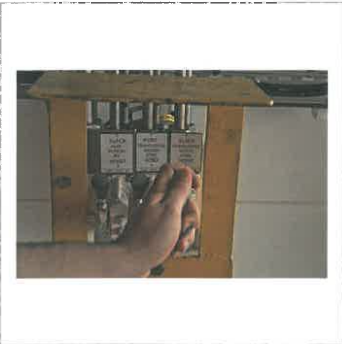
Spread rope winch #1 control
