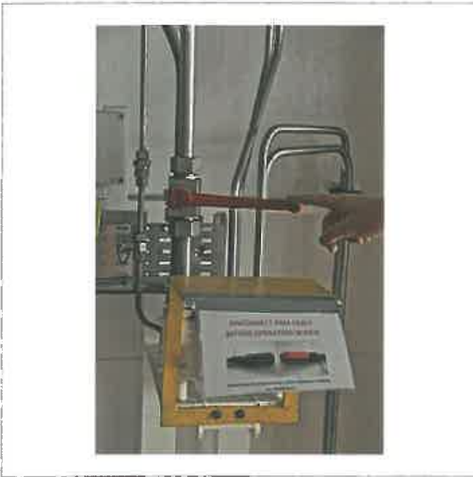
Hydraulic shut-off valve (in off position)
