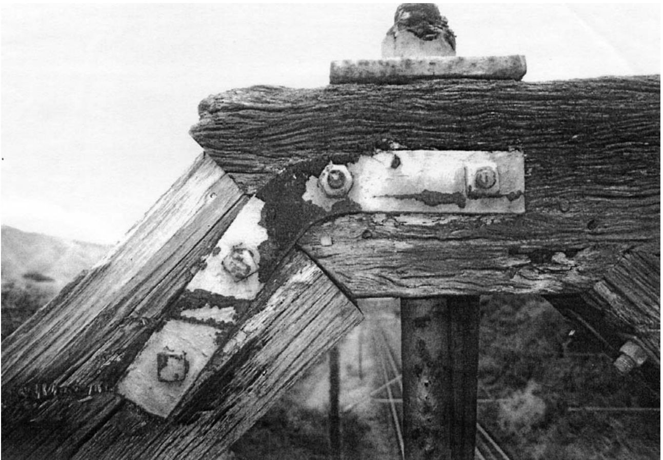
Fig. 12: Fish plate joining top chord with end strut on a Howe truss. Pukerua Bay road bridge over NIMT.
