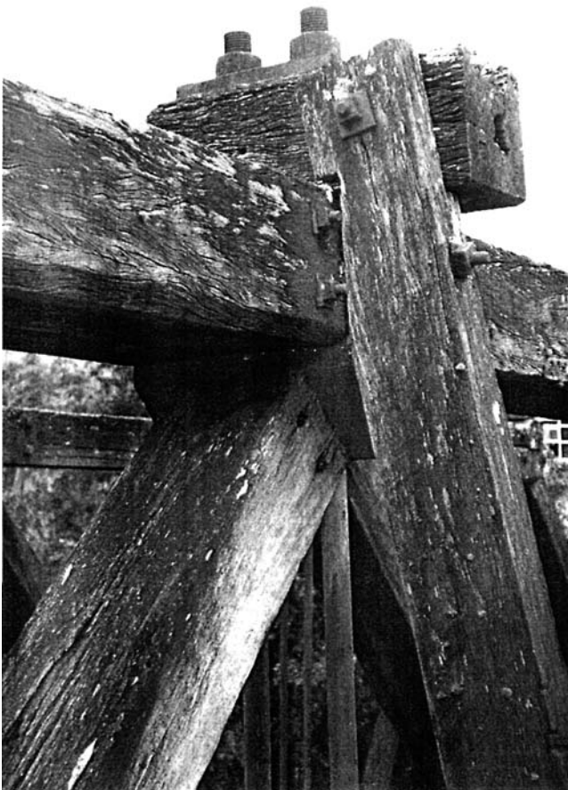
Fig. 23: Top chord and associated timbers on Waikino rail bridge. Note pipe rot on saddle block, upper end grain rot on truss brace. A rainproof cap would have prevented this.
