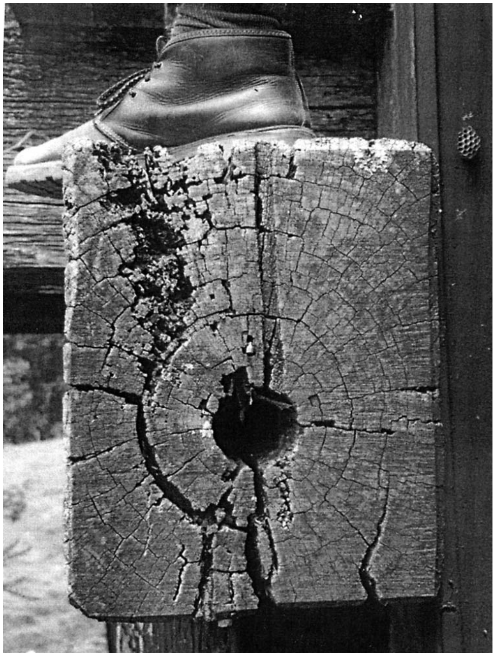
Fig. 16: Pipe rot in 'boxed heart' beam. Bridge on Waihi goldfields railway.
