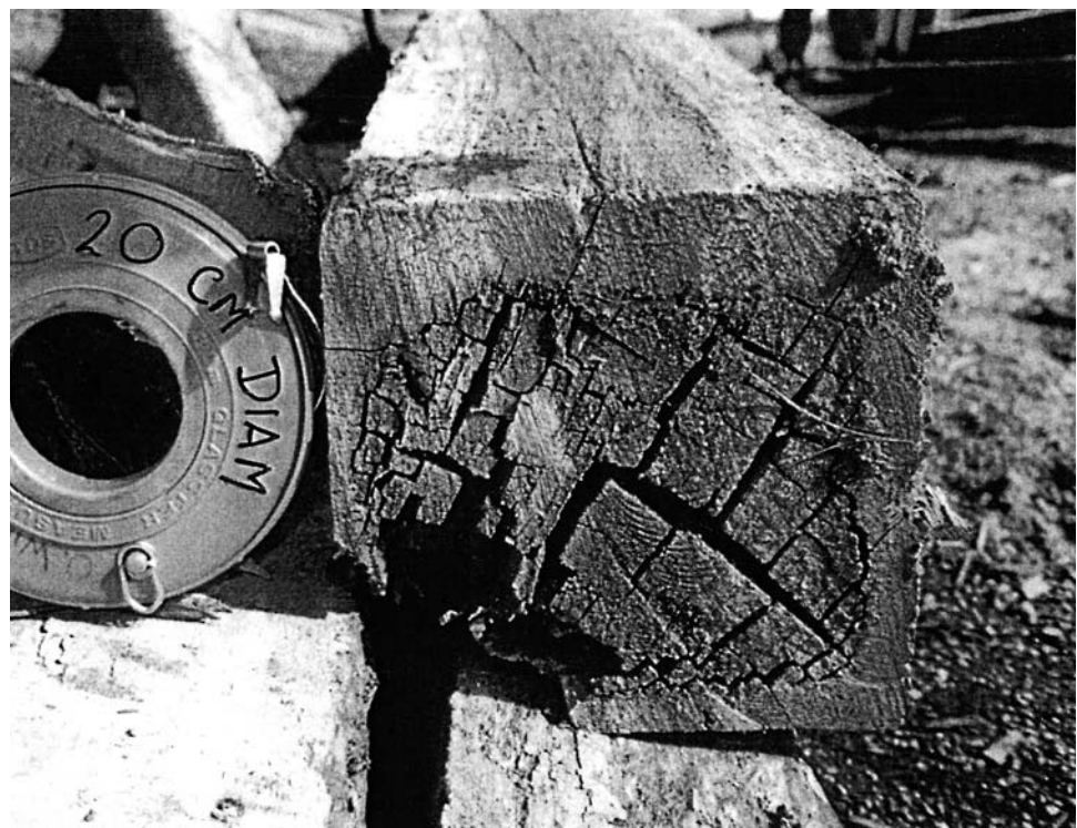
Fig. 8: A bad case of internal rot in kauri from suspension bridge tower in the Kauearanga valley. This rot was not evident until the post was cut down.
