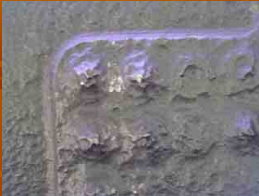
Lifting chain damage to coating
