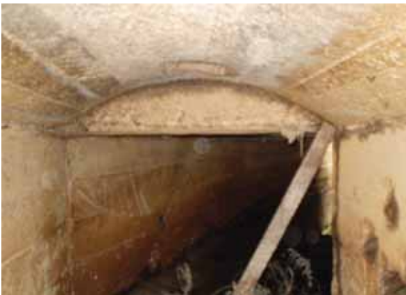
Inside the fanhouse drainage tunnel. Top: looking towards the Capell fan foundations. Below: showing the diagonal brace that impedes some material. JOHN OLIVER
