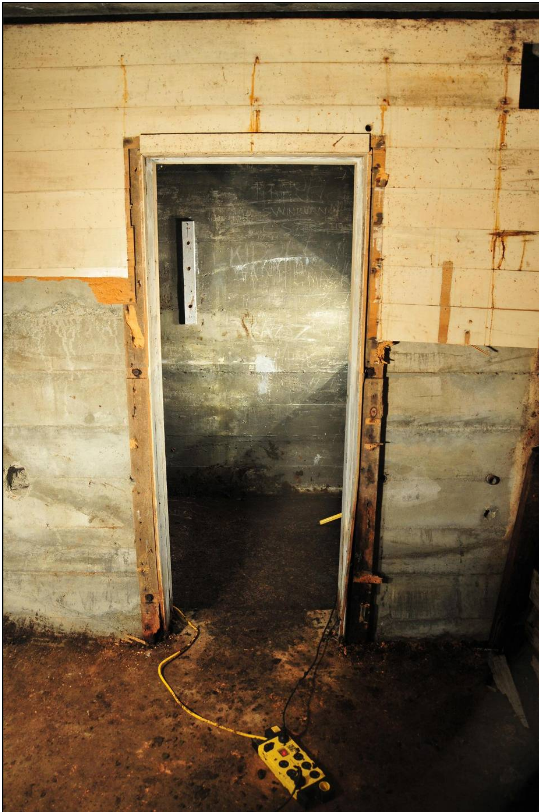
Appendix 5: The doorway of the radio room. Shows the painted timber overlaid on concrete walls (DoC).
