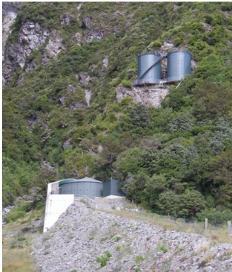
Figure 3 – Fire-fighting tanks (top), header tank, balance tanks and treatment plant (bottom), Glencoe Stream.
