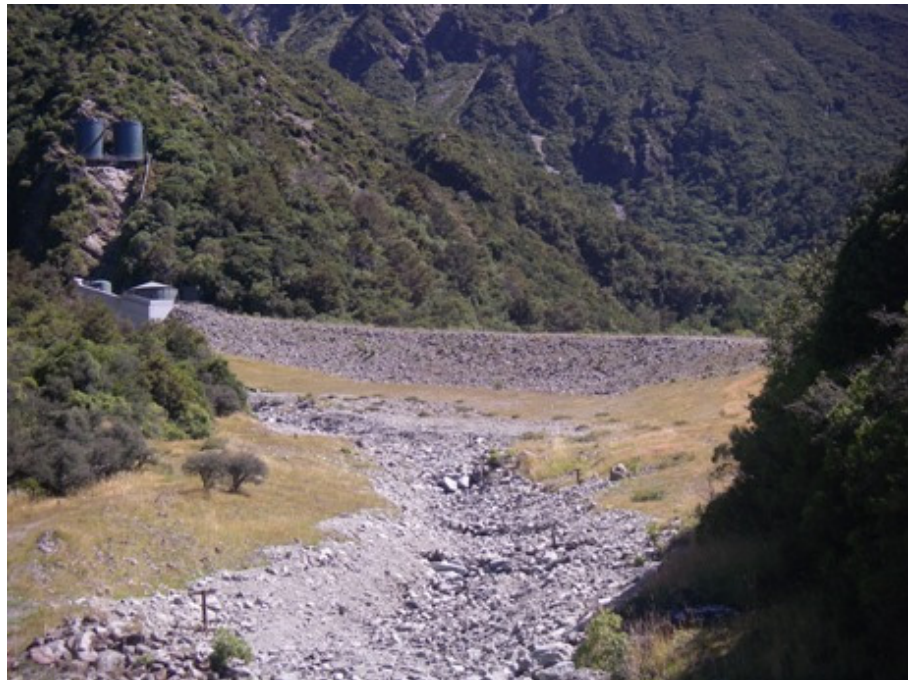
Figure 11 – Glencoe Stream flood protection – rock stop banks and concrete training wall (left).
