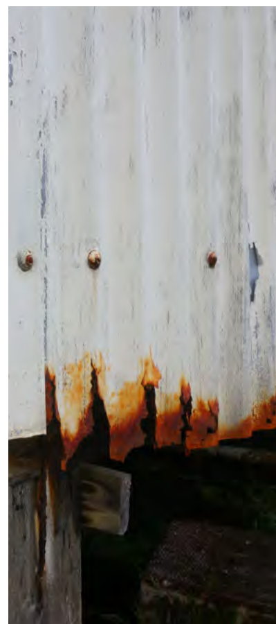
Figure 1-19 ABOVE Cladding corrosion at the base of a wall.
