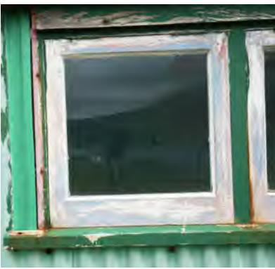
Figure A5 ABOVE -The south window, in poor condition. This will be leading to leaks and the high moisture content (27%) below this window.
