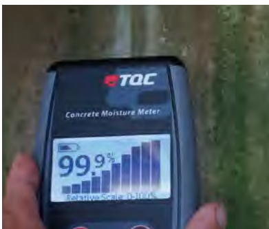
Figure L11 BELOW Moisture readings in the meat outhouse, showing complete water saturation at 99.9% out of 100%. Readings inside a building should be between 30% & 40% typically.
