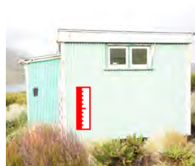
Figure A1 ; A2 ; A3 ; A4 The four elevations of Aurora Hut. The patches are where the plastic cladding, added over the previous, have cracked and deteriorating. The timber cladding below was leaking before the plastic over-clad.
