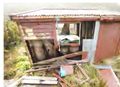
Figure 1-1 ABOVE The very historic Tucker Hut, near to demolished by neglect.
