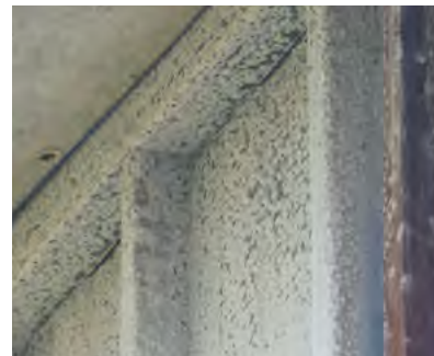
Figure 1-14 ABOVE The upper area of the cladding on the accommodation buildings, where zinc has extensively oxidised. The next stage of the corrosion cycle is perforation.
