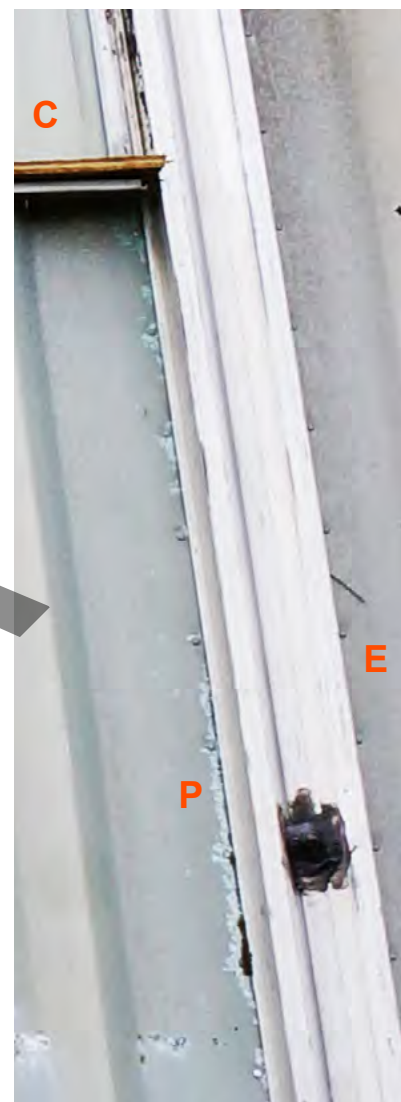
Figure 1-12 Corrosion evident on the left hand side, where the copper treated shutters have been added above. The aluminium is in pristine condition for its age on the right hand side where there was no treated copper shutters added above.
