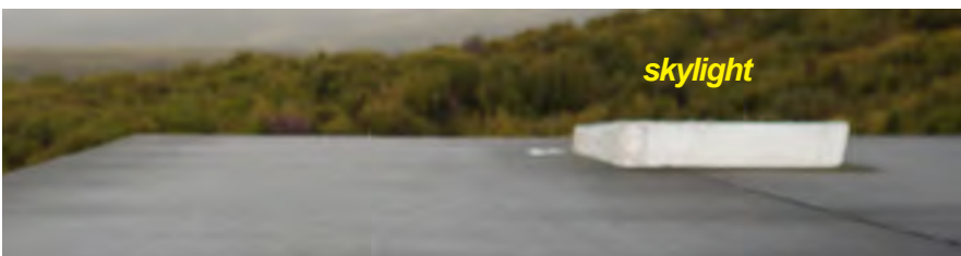
Figure A8 ; A9 ; A10 The roof membrane is in good condition, but very poor detailing around all the edges means that the roof will leak &/or peel off in high winds. The skylight has no upstand and this will lead to inevitable decay if no corrective action is completed.
