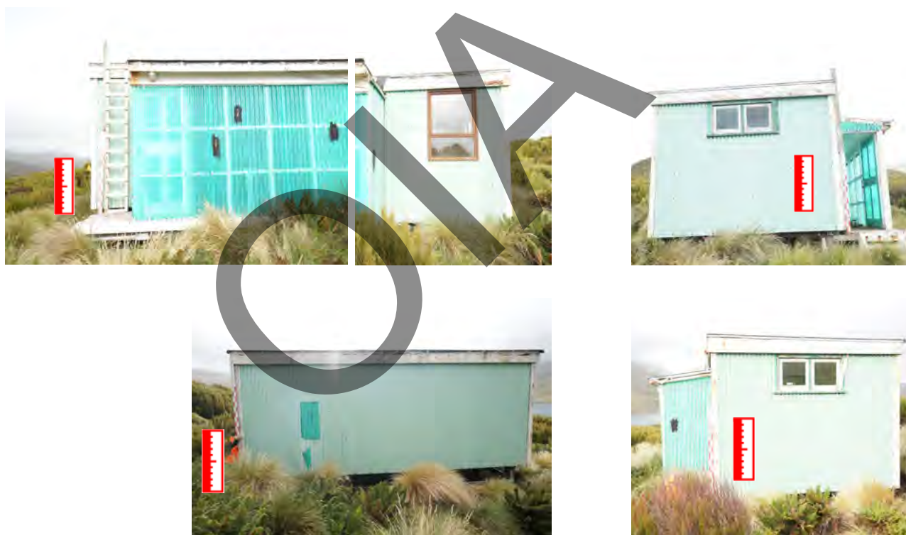
Figure A1 ; A2 ; A3 ; A4 The four elevations of Aurora Hut. The patches are where the plastic cladding, added over the previous, have cracked and deteriorating. The timber cladding below was leaking before the plastic over-clad.
