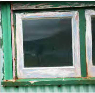
Figure A5 ABOVE -The south window, in poor condition. This will be leading to leaks and the high moisture content (27%) below this window.
