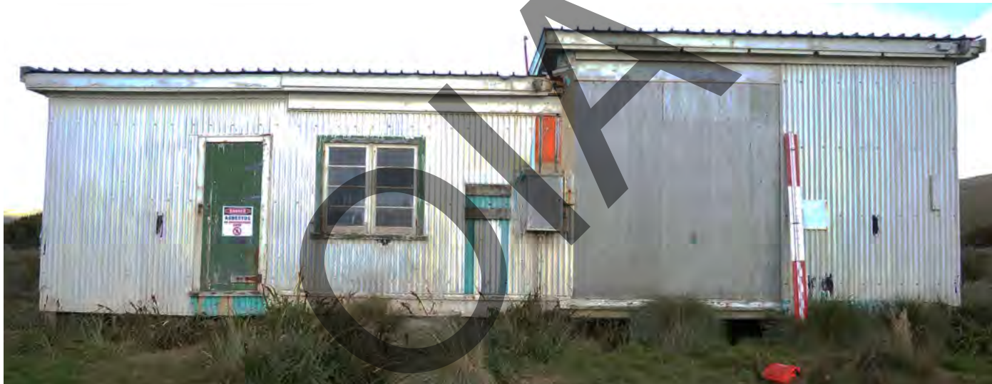
Figure 1-7 ABOVE The historic hydrogen building, near to demolished by neglect
