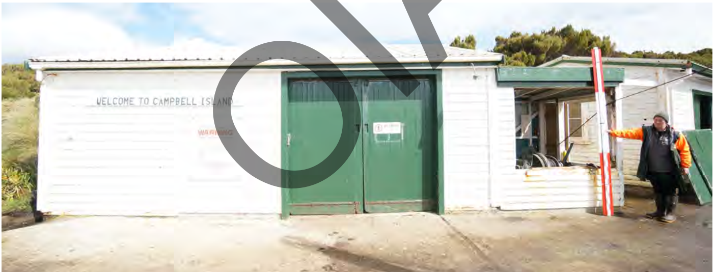
Figure S1 BELOW East elevation of Jetty Store with winch alcove, with window openings removed and on the ground leaning against the Spirits / Paint store.
