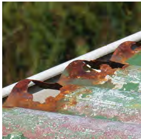
Figure N8 BOTTOM RIGHT Rust starting in areas of the original cladding not replaced.
