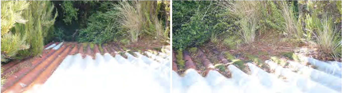
Figure L7 ; L8 ; ABOVE. Simple house keeping measures, which involves the removal of moss and forest litter from the roof, would allow the roofing to dry and would remarkably extend the durability of the roofing.
