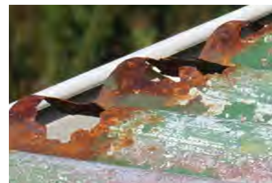
Figure 1-6 ABOVE A lot of the cladding around Beeman Base is ending its natural life. In this case the roofing has perforated.
