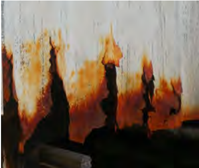
Figure 1-9 ABOVE Corrosion on ferrous cladding material, installed post 1960,
