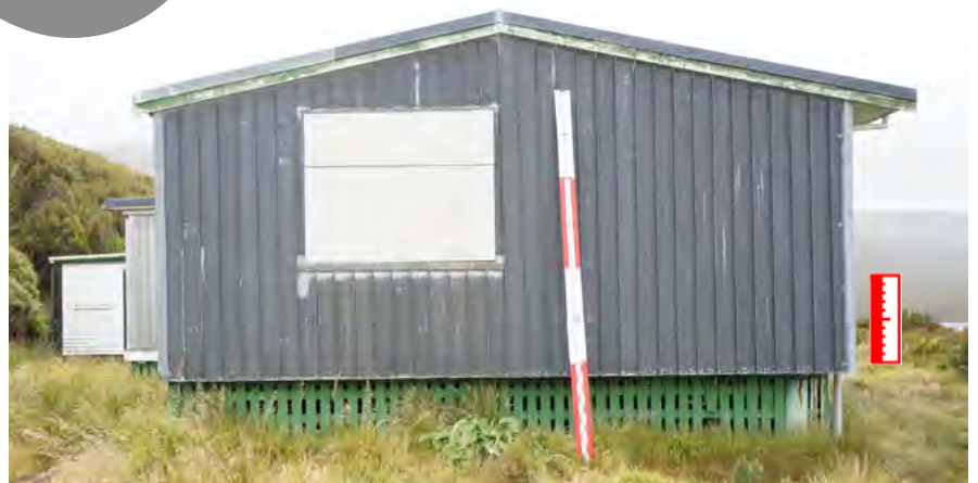
Figure H3 ABOVE The recent zinc clad addition at the south end of the Hostel. The copper treated shutter installed over the window shown in this photo is corroding the zinc.
