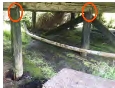
Figure 1-8 BELOW The typical structure, minor modifications required to add connections to limit earthquake damage are missing, red circle.
