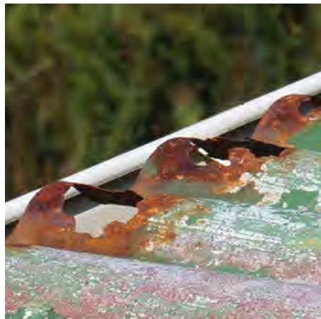
Figure N8 BOTTOM RIGHT Rust starting in areas of the original cladding not replaced.
