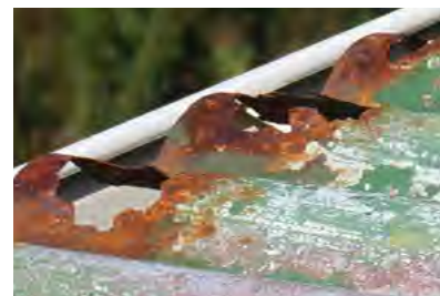
Figure 1-6 ABOVE A lot of the cladding around Beeman Base is ending its natural life. In this case the roofing has perforated.
