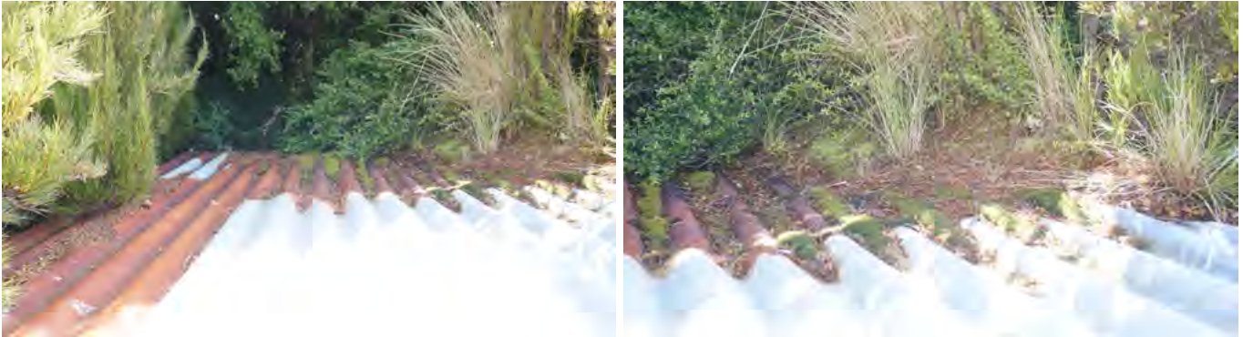
Figure L7 ; L8 ; ABOVE. Simple house keeping measures, which involves the removal of moss and forest litter from the roof, would allow the roofing to dry and would remarkably extend the durability of the roofing.
