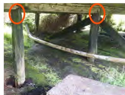
Figure 1-8 BELOW The typical structure, minor modifications required to add connections to limit earthquake damage are missing, red circle.
