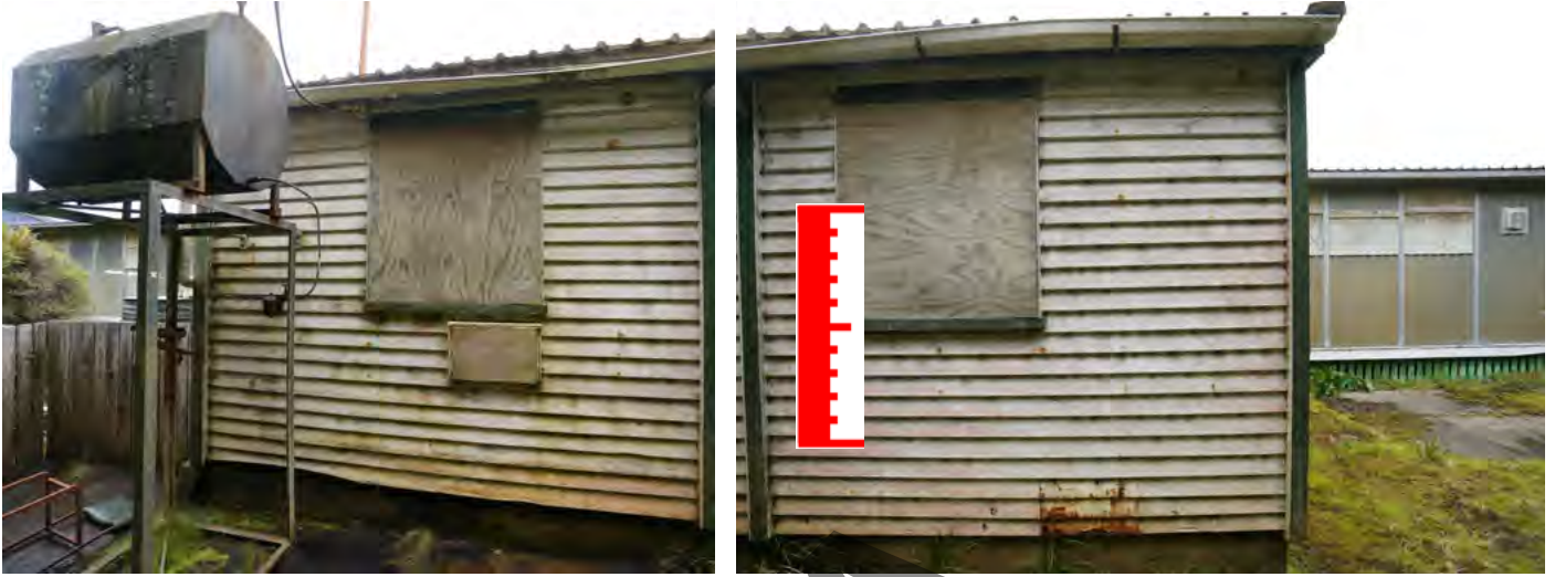
Figure H6 & H7 ABOVE The west elevation of the Hostel, the west wall of the store.
