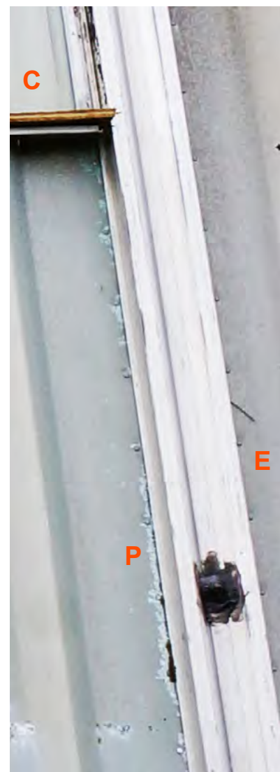
Figure 1-12 Corrosion evident on the left hand side, where the copper treated shutters have been added above. The aluminium is in pristine condition for its age on the right hand side where there was no treated copper shutters added above.
