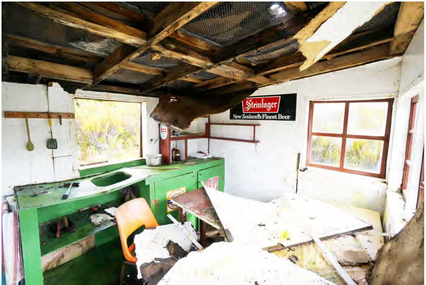
Figure V7 BELOW The ceiling has collapsed onto the furniture below. Holes in the roof are visible as light patches. The window is missing. The towel in the far left bottom corner has remained relatively clean with all the internal moisture.
