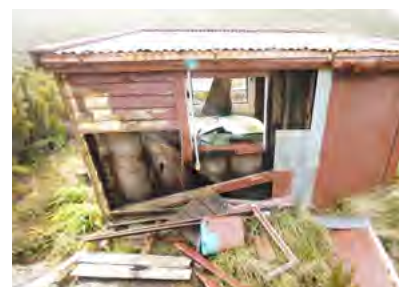
Figure 1-1 ABOVE The very historic Tucker Hut, near to demolished by neglect.
