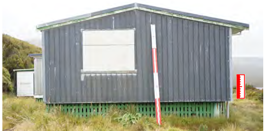
Figure H3 ABOVE The recent zinc clad addition at the south end of the Hostel. The copper treated shutter installed over the window shown in this photo is corroding the zinc.
