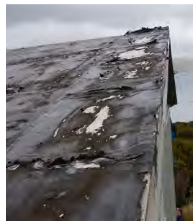
Figure T12 ABOVE The original aluminium clad roof, with a membrane over, an economical possible solution to remedy the roof leaks. This membrane is now ending its effective life.
