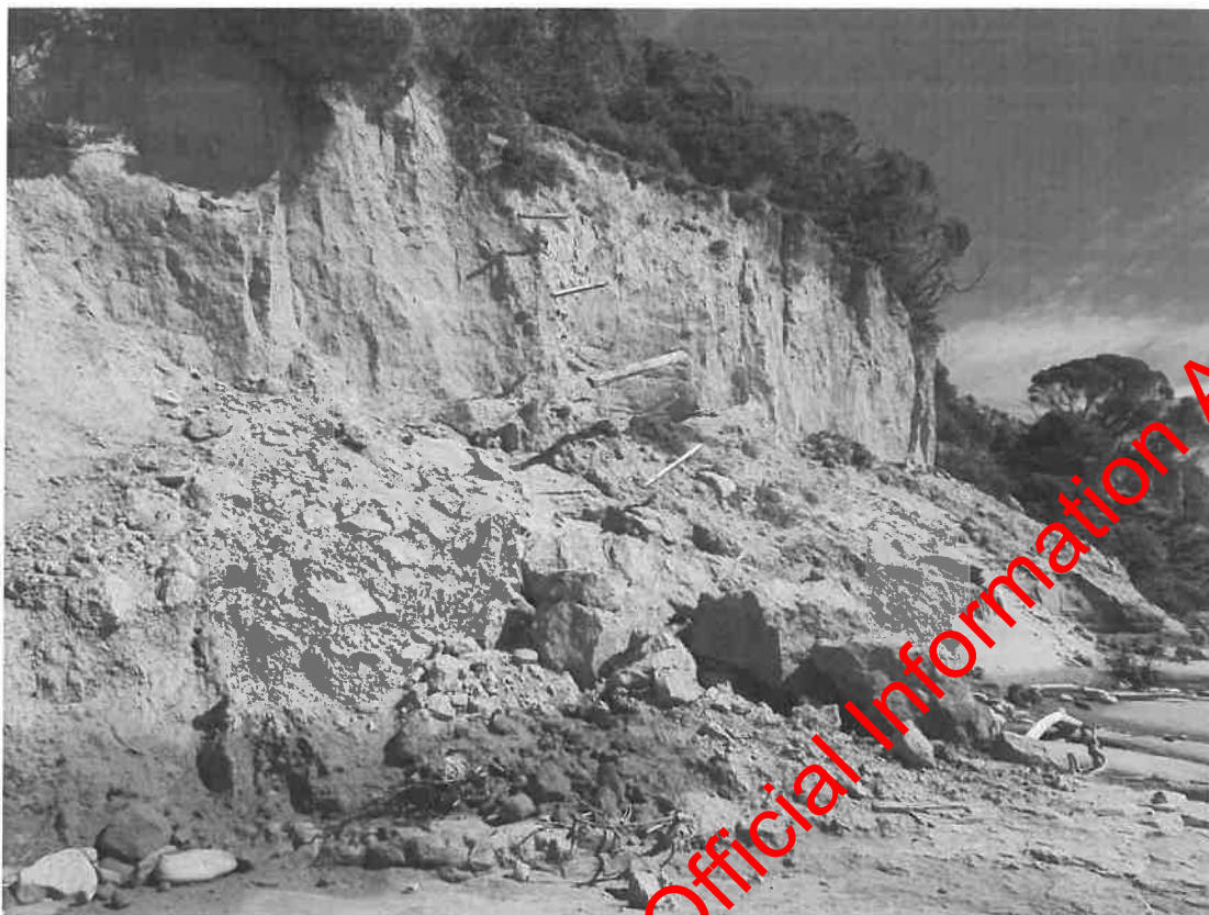
Image 4 Example of hanging fenceline that has been subject to the eroding cliff line
