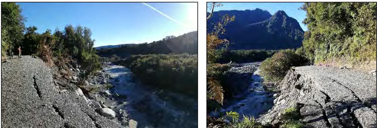
Figure 1-9 – Photos of the South Washout 2 location – looking downstream & upstream
