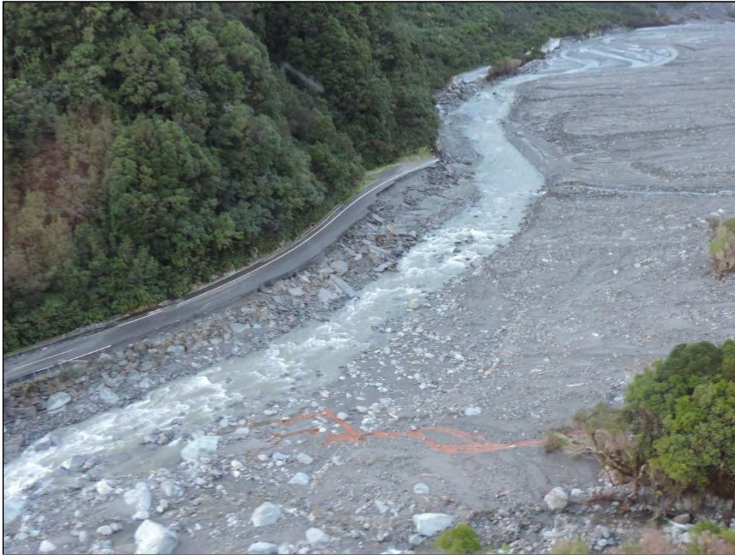
Photo 21 - North Washout 2, looking upstream.
