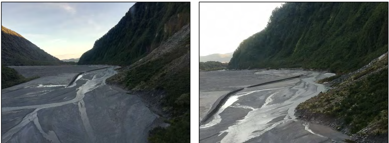
Figure 1-7 – Photos of the upper section of the road, now destroyed – looking downstream
