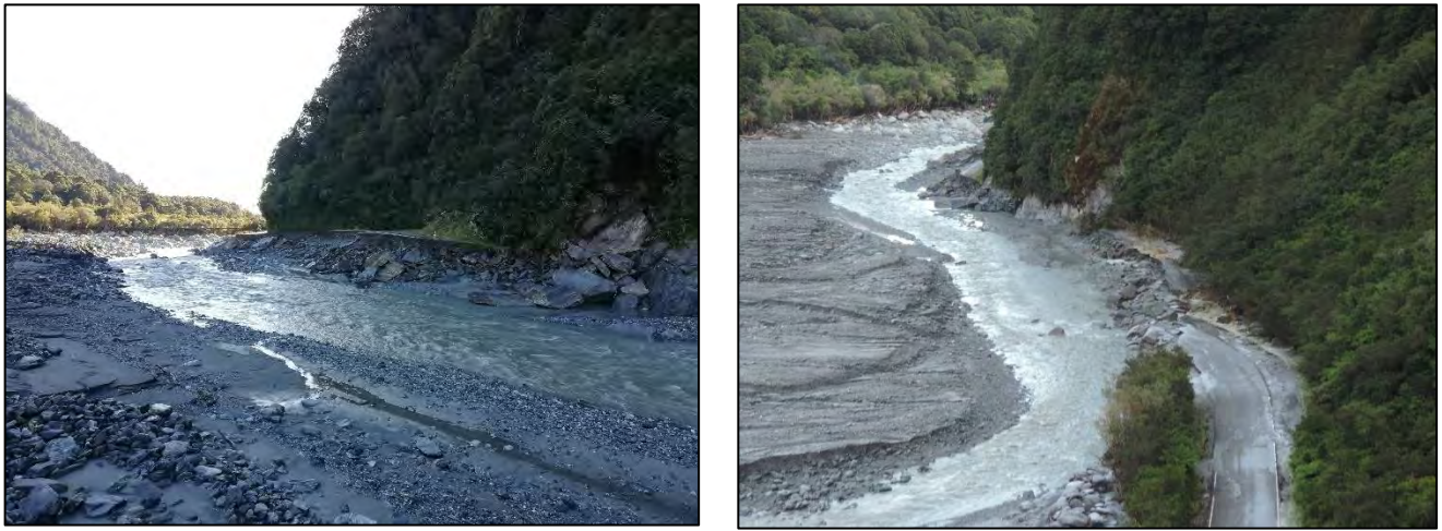
Figure 1-6 – Photos of the North Washout 3 location – looking downstream
