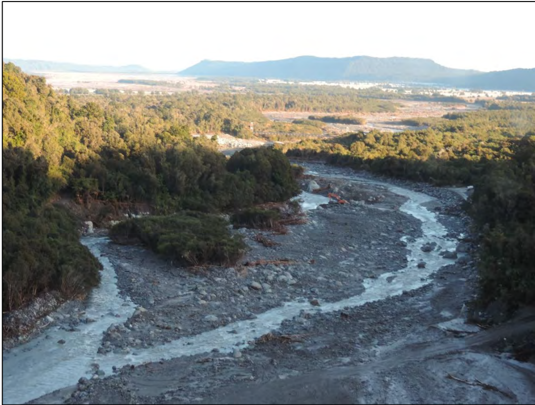
Photo 27 - The channel splitting that has developed along the river reach. The South Washout 2 is on the left side at the point of the island where there is remaining vegetation. The old dump is on the right side, opposite where the excavator is working.
