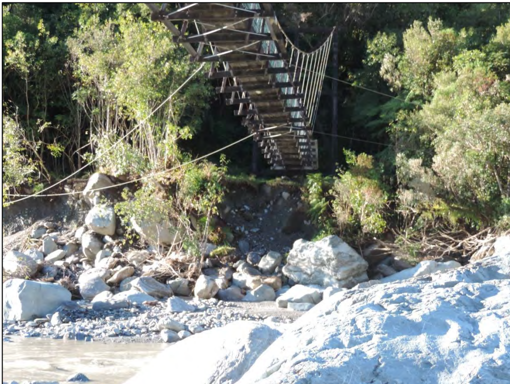
Photo 16 - A closer view of the right side, with the bridge tower on a concrete footing just above the raw bank that can be seen underneath the bridge.
