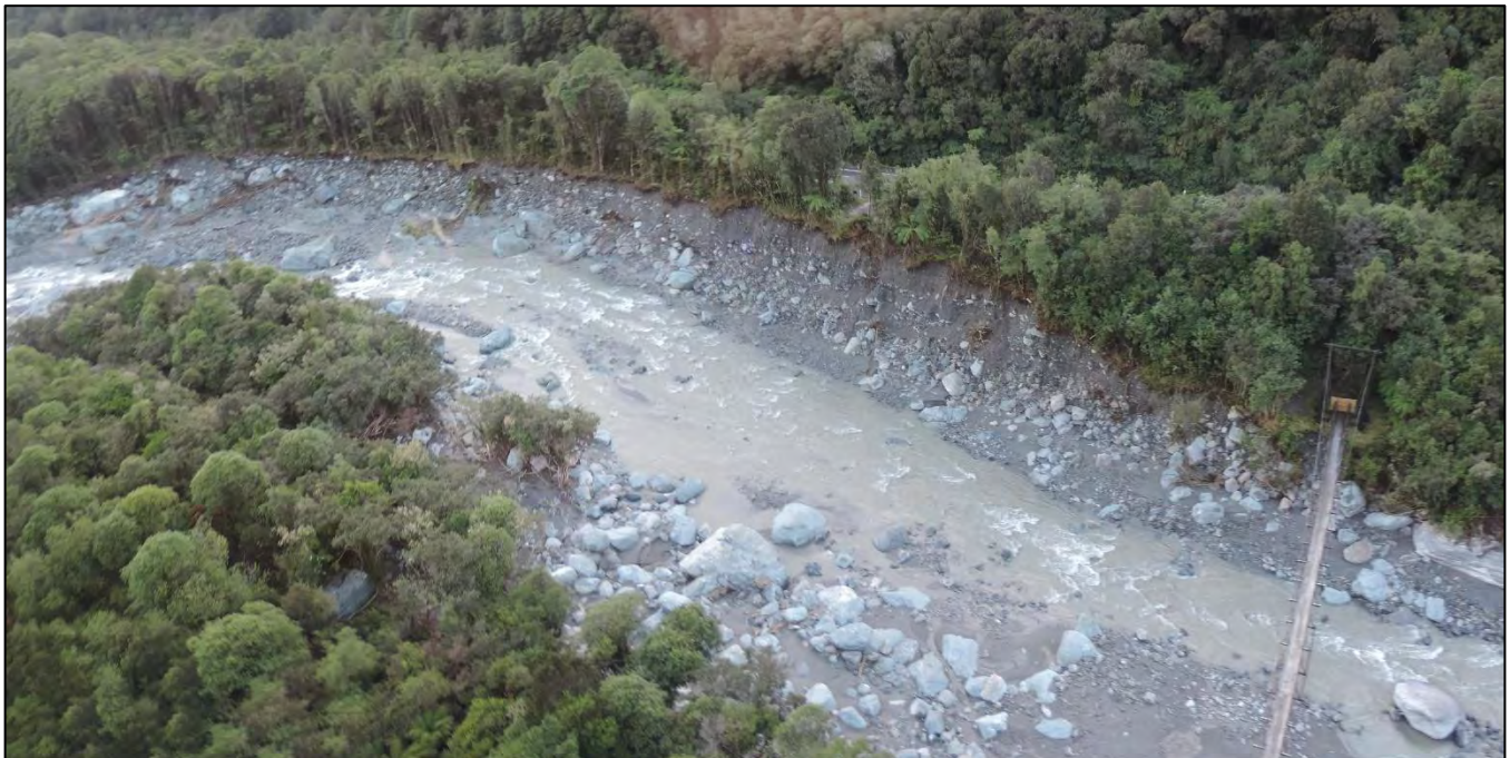
Figure 3-1 – Erosion embayment at and downstream of bridge
