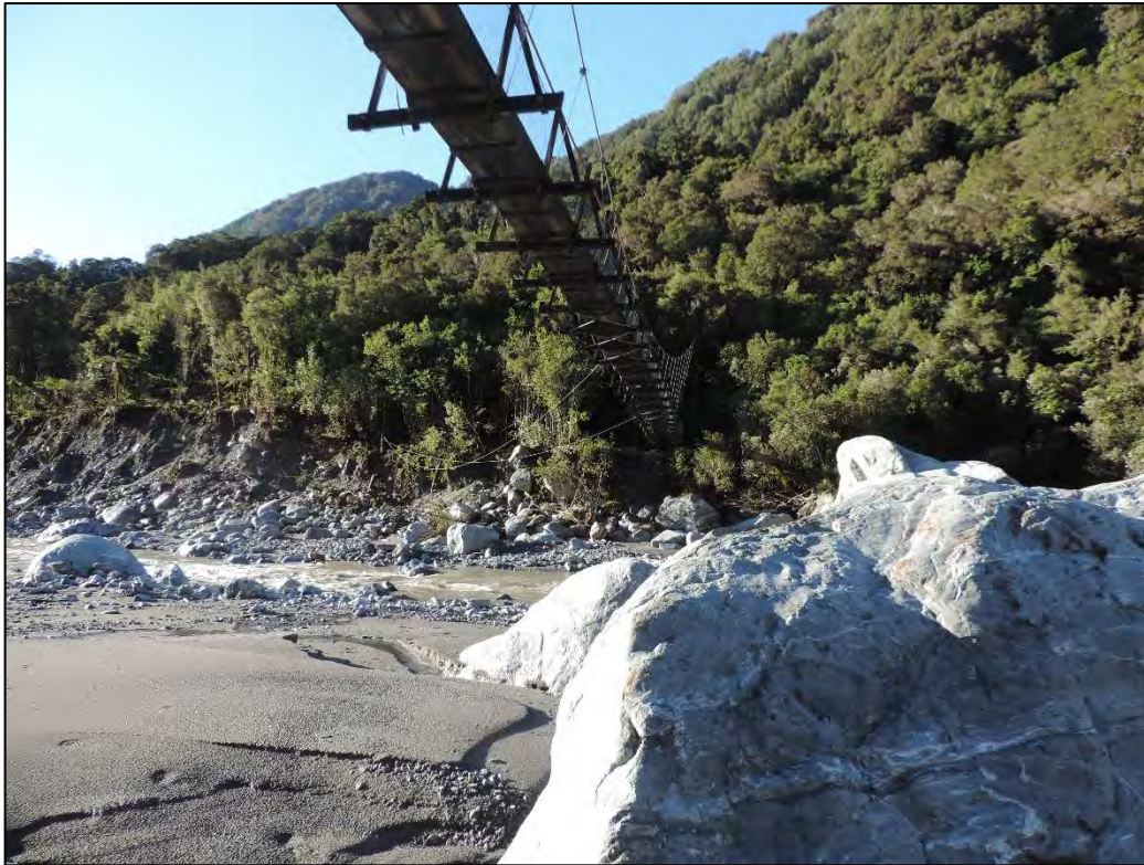
Photo 15 - The right (north) side of the abutment, showing the eroding bank, with a large boulder in the foreground.
