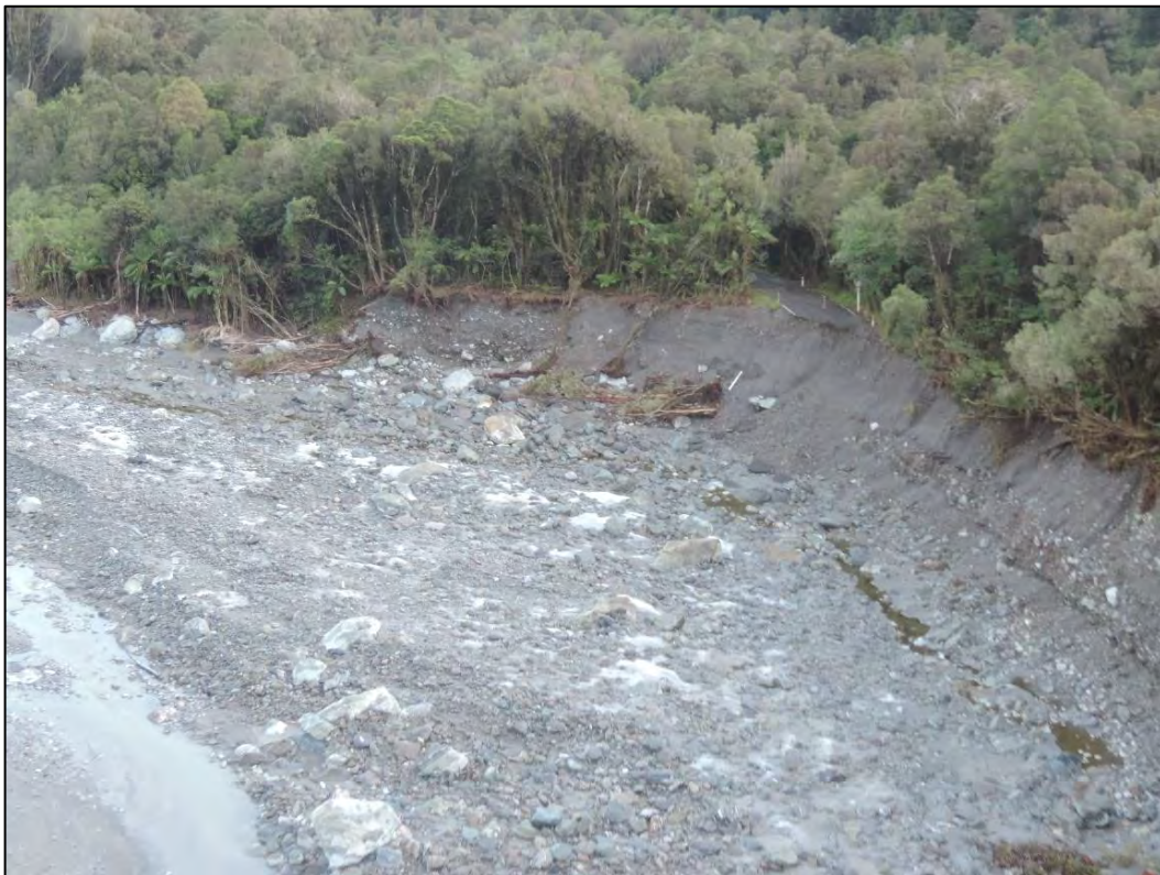
Photo 26 - The erosion embayment that gave rise to the North Washout 1. Note the road on the bank crest, where there is a square shadow. Note also the fineness of the river bank material compared to the river bed.
