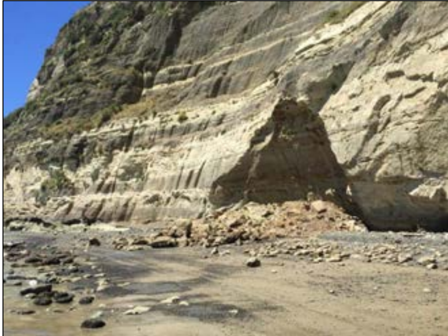
Figure 3-14: Sector 5 - an example of recent landsliding triggered by erosion at the toe of the slope
