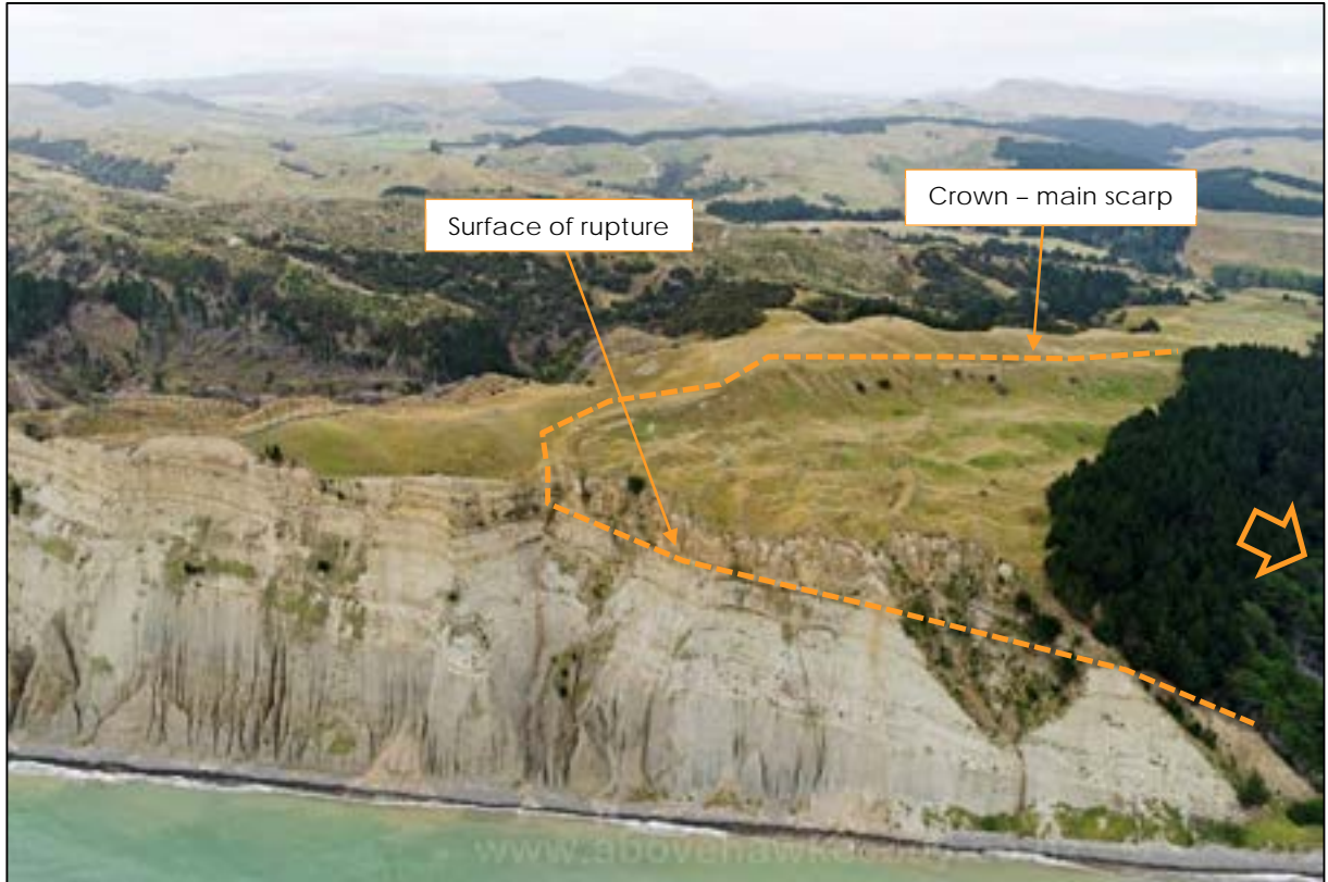
Figure 4-9: Sector 1 - A large deep-seated landslide, where the surface of rupture appears to be along bedding
