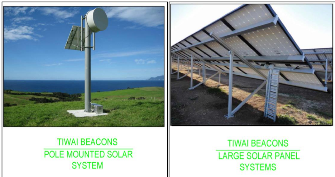
Figure 1-3 Examples of pole mounted solar system and large solar panel system.
