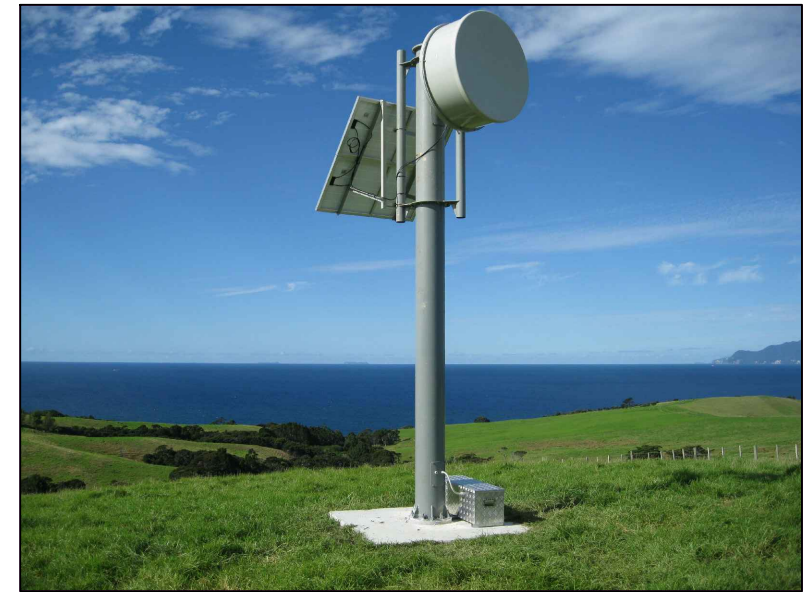
TIWAI BEACONS POLE MOUNTED SOLAR SYSTEM
