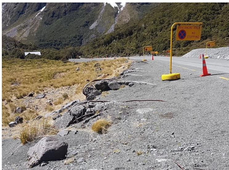
Photo 12: remnant steel and concrete from 1960s avalanche protection shelter demolished by avalanche in 1960s.
