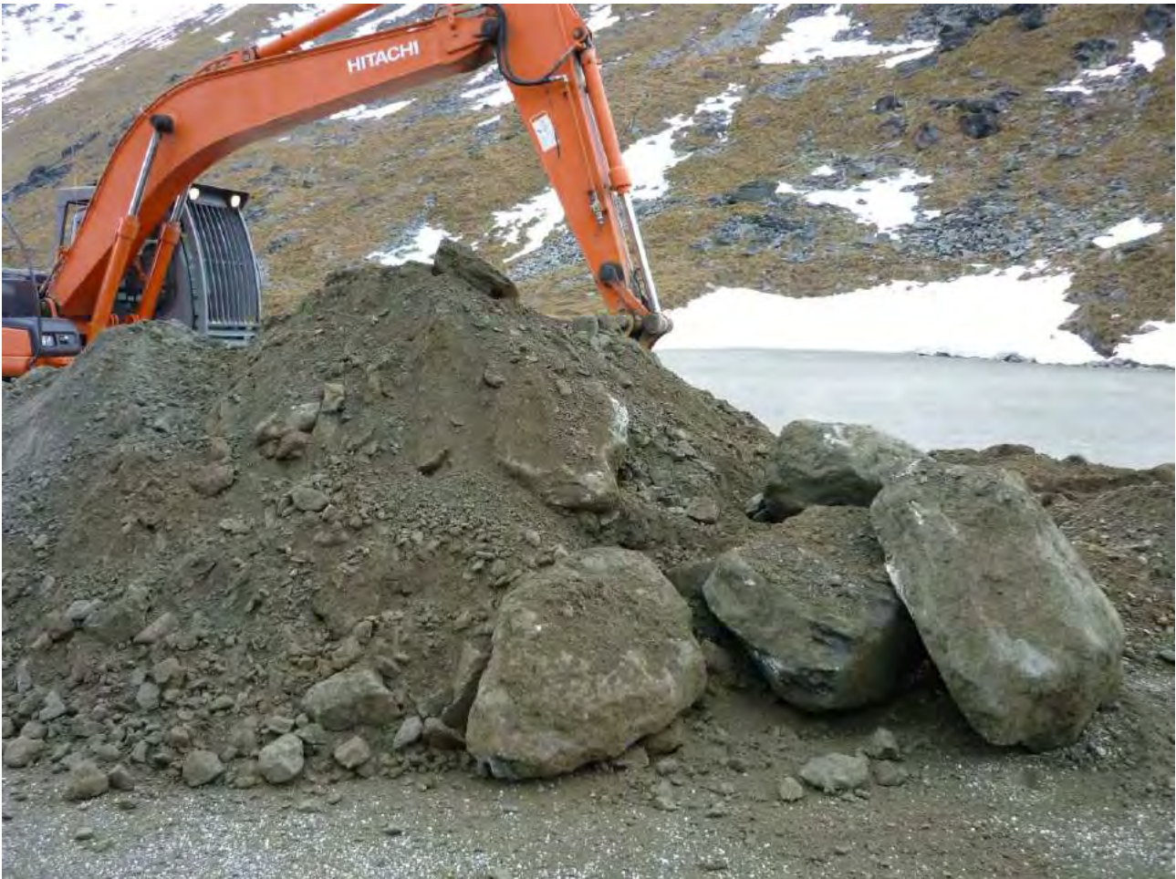
Figure 5-1: test pit excavation at the base building site in undisturbed dense glacial till
