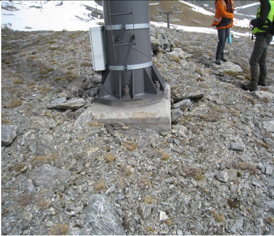
Figure 15: Example of tower to be removed as part of decommissioning Sugar Bowl chairlift (Photo 031)
