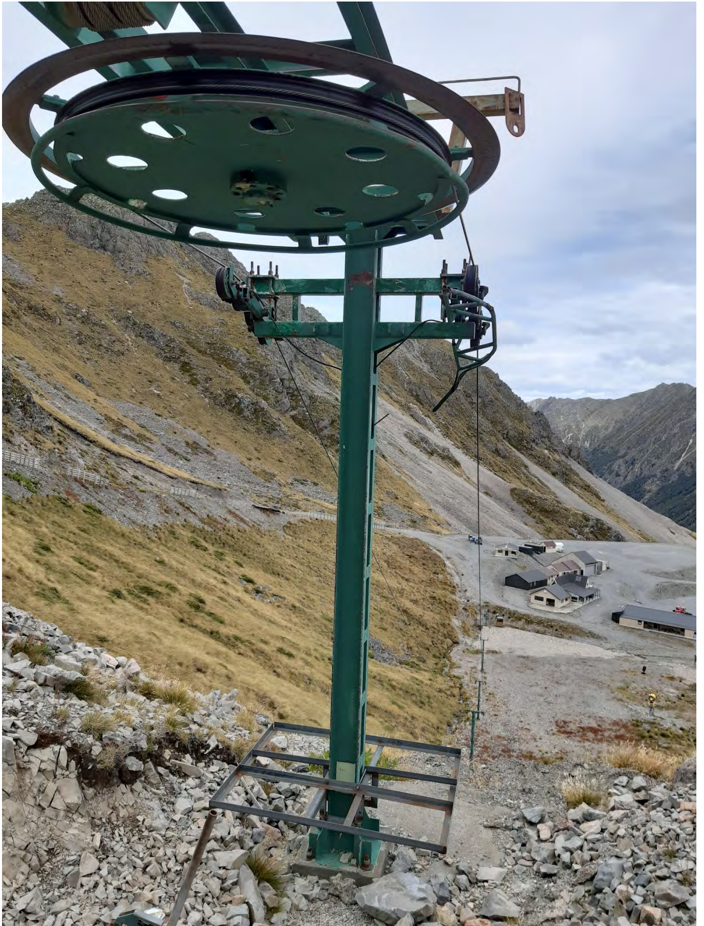
Figure 45: Platter lift top tower looking down to the drive terminal
