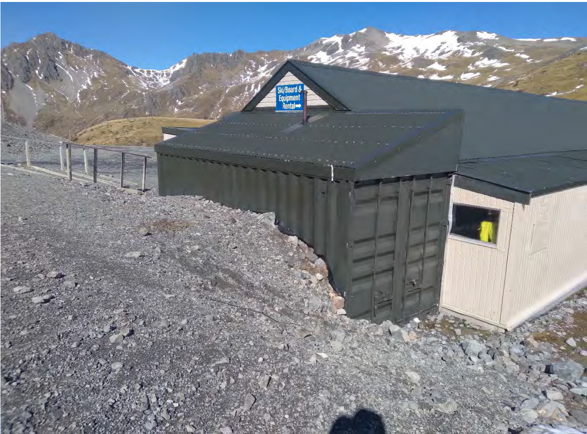
Figure 20: Generator shed 100KVA
