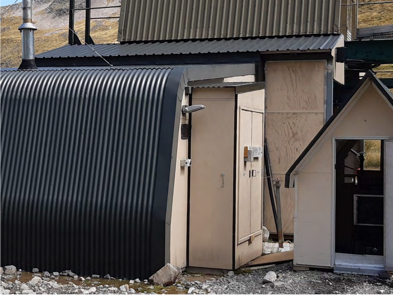
Figure 77: Fuel bowser on side of 300KVA generator shed
