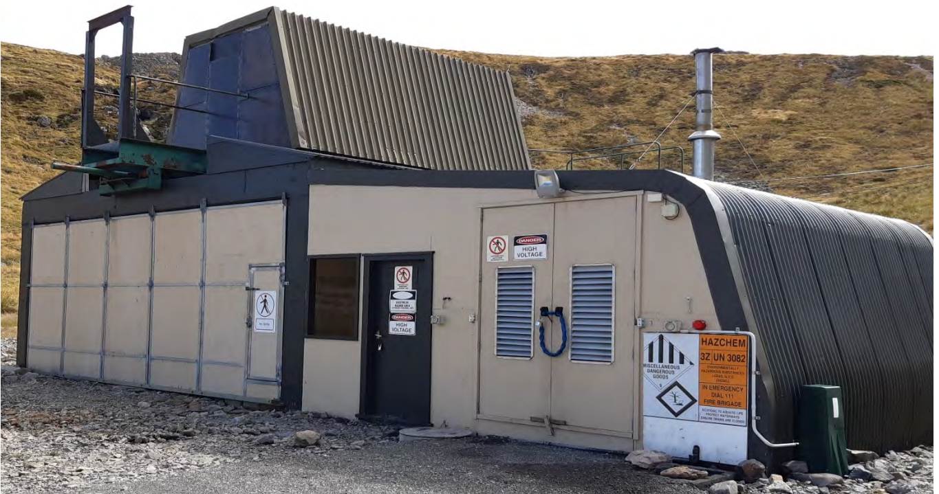
Figure 33: T-bar drive terminal and 300KVA generator shed
