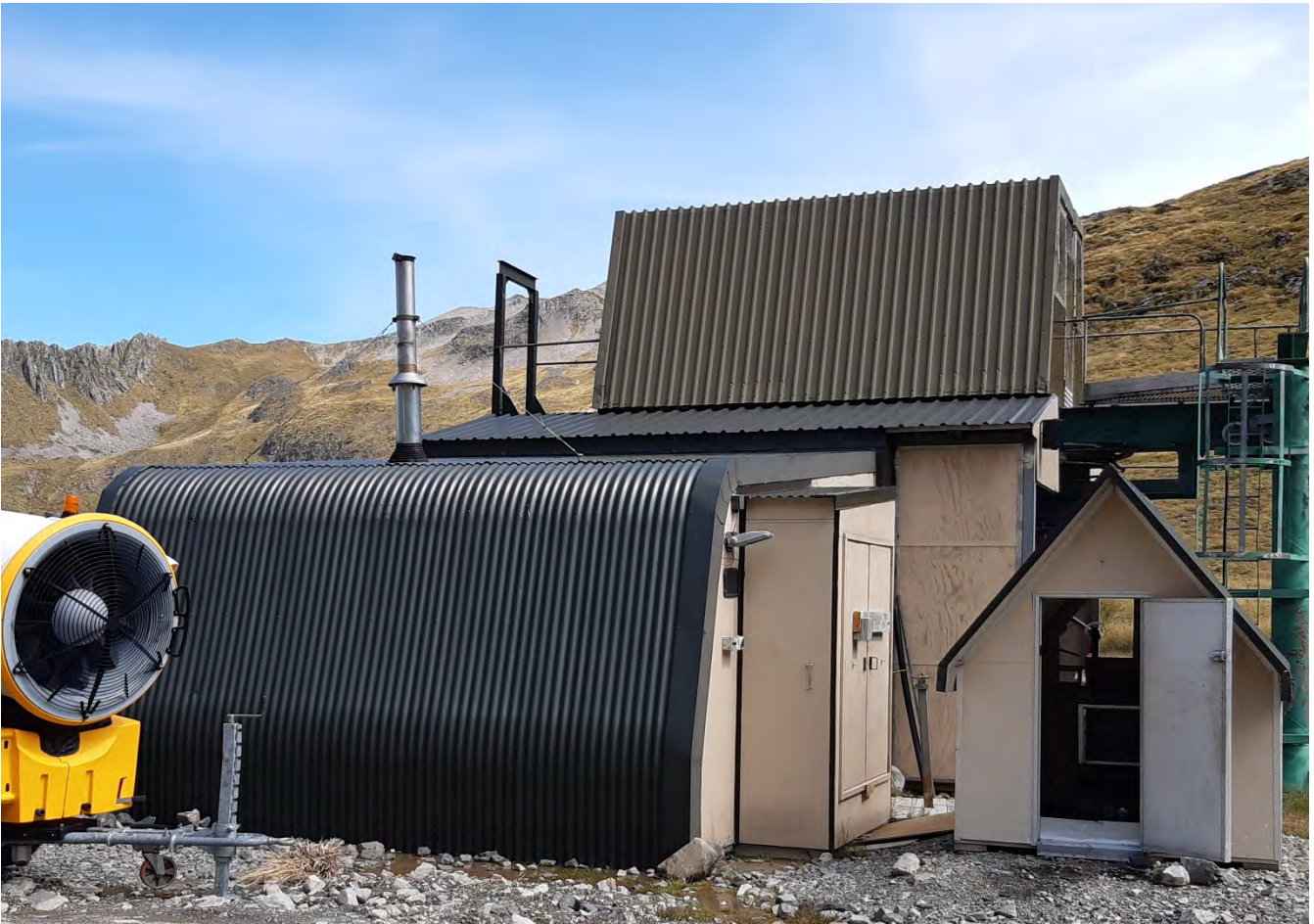
Figure 34: Generator 300KVA and 17KVA
