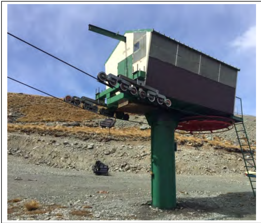
Figure 2 T Bar Drive Station
