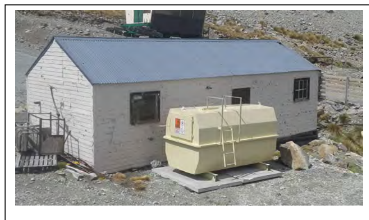
2000 litre bunded diesel storage tank
