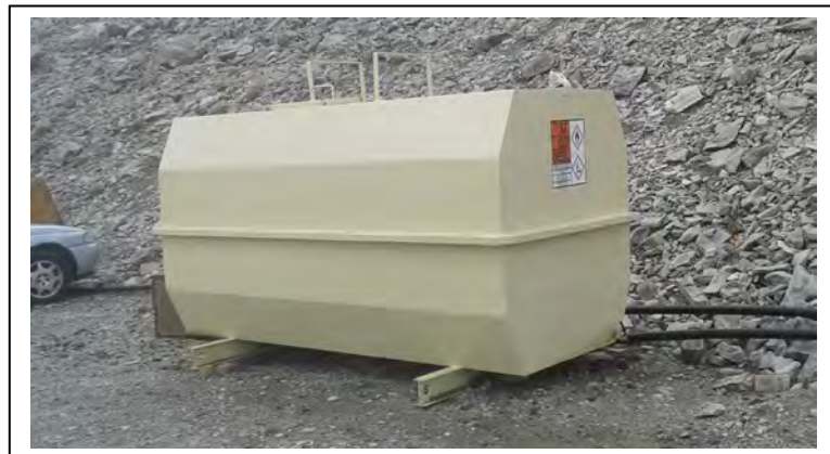
2000 litre bunded diesel storage tank
