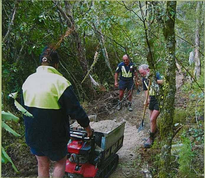
The team using a motorised wheelbarrow to lay pumice on the new track. Photo: Kim Alexander/aria
