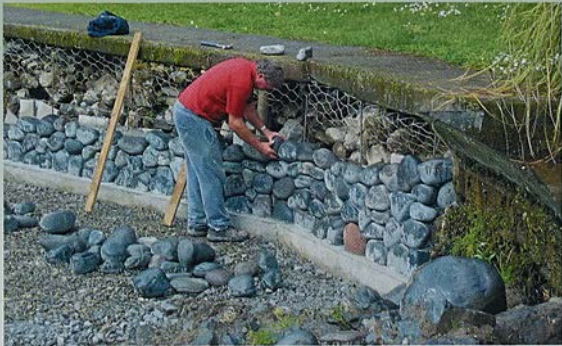
Gurdon Hydes places the rocks as the new wall begins to take shape. Photos: Errol Cudby
