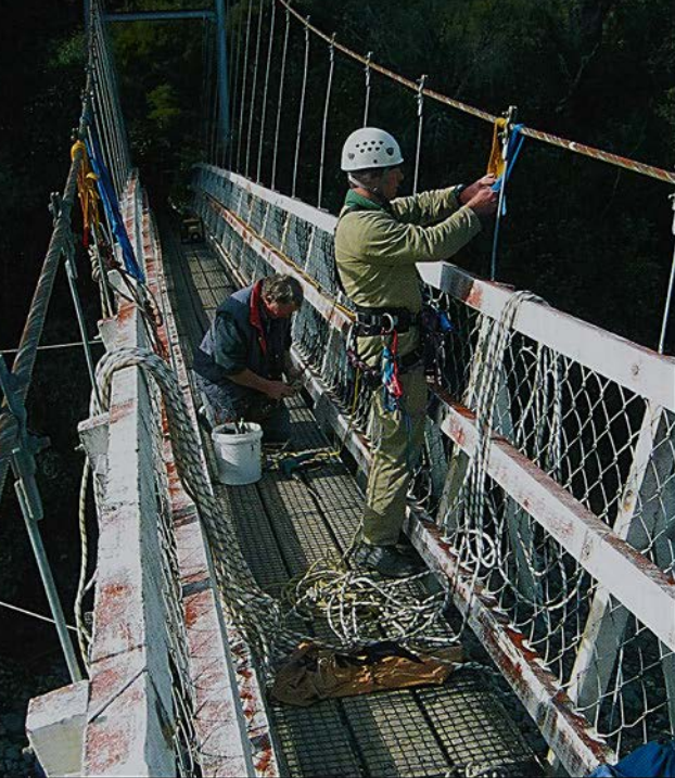
A flood-borne pine tree also caused minor damage to the Red Hut foot bridge. Rob Kirkwood and Gordon Hyde get ready to undertake repairs. Photo: Dave Hart
