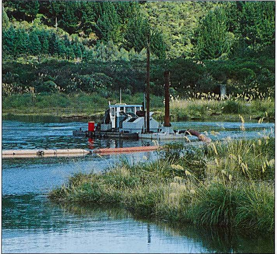
The cutter suction dredge in operation in Lake Te Whaiau just upstream of the road bridge
