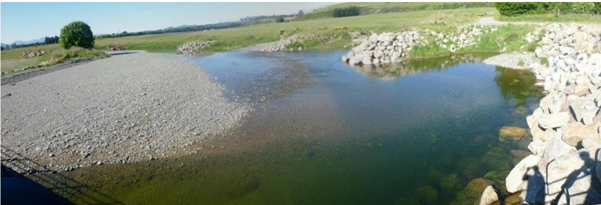
Photo 3: constructed groynes in 2014 with gravel beach build up on true right side of River (left of photo).
