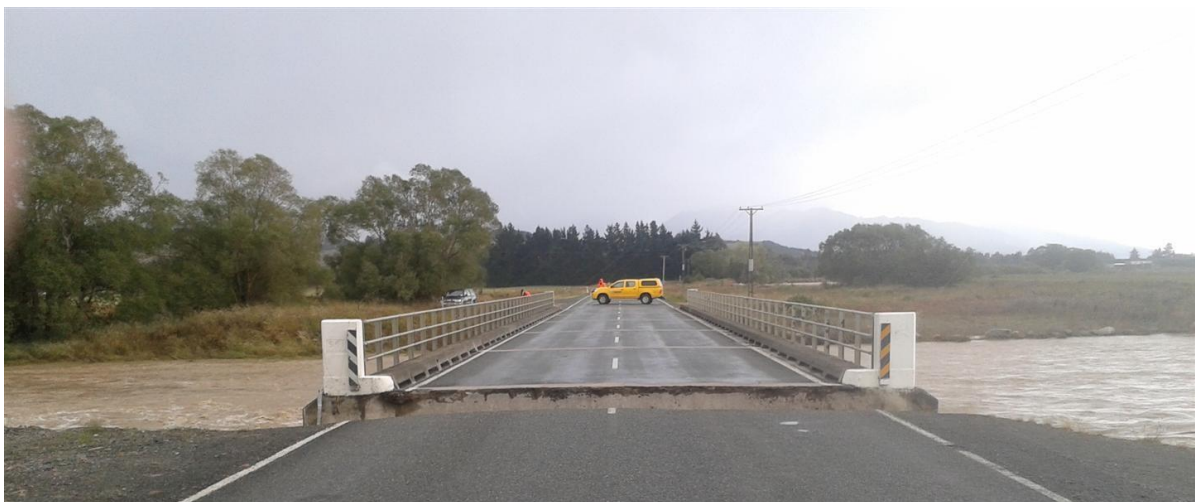
Figure 2: Photo of Whitestone River (SH 94) Bridge Washout taken January 2013
