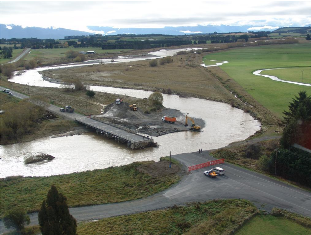
Photo 1: SH94 Whitestone River Bridge approach washout in April 2010.
