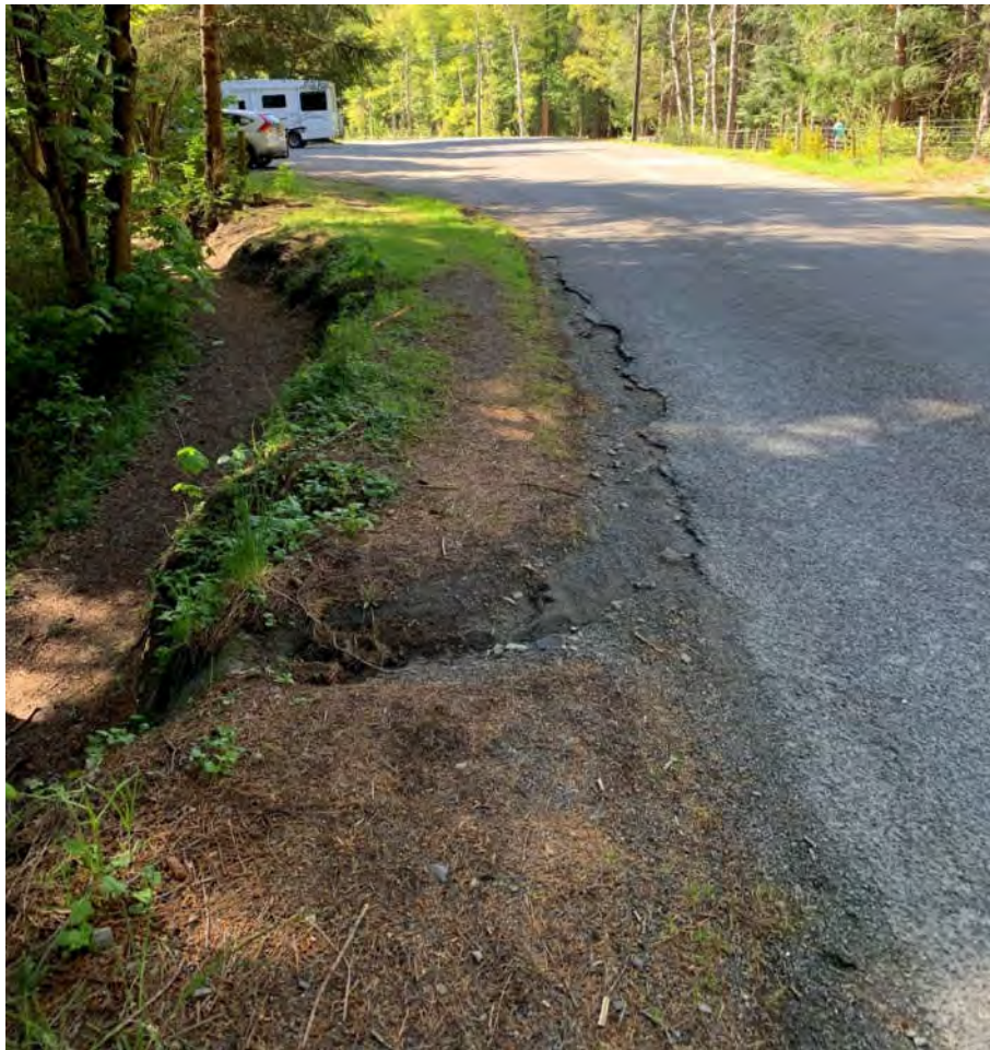
Photograph 12: Track Along the Edge of the Road Shows Potential Water Damage (Edge of Seal and Culvert Location)
