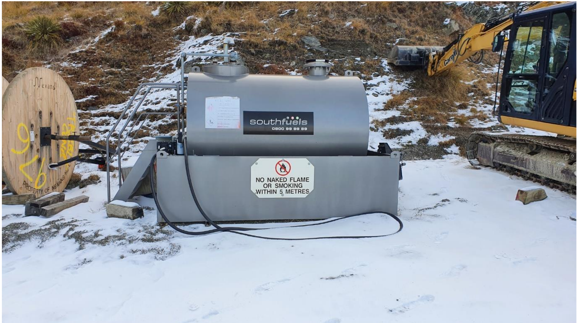
Figure 23 Bulk Fuel Storage – Petrol
