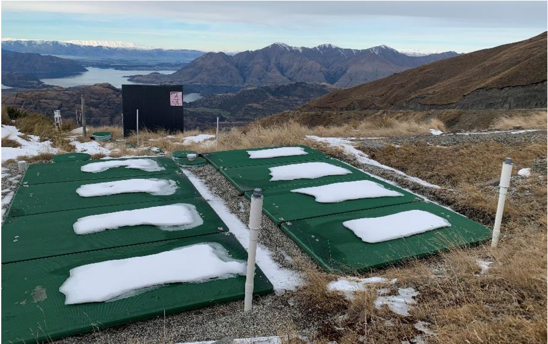
Figure 31 Wastewater Treatment Plant incl pump shed
