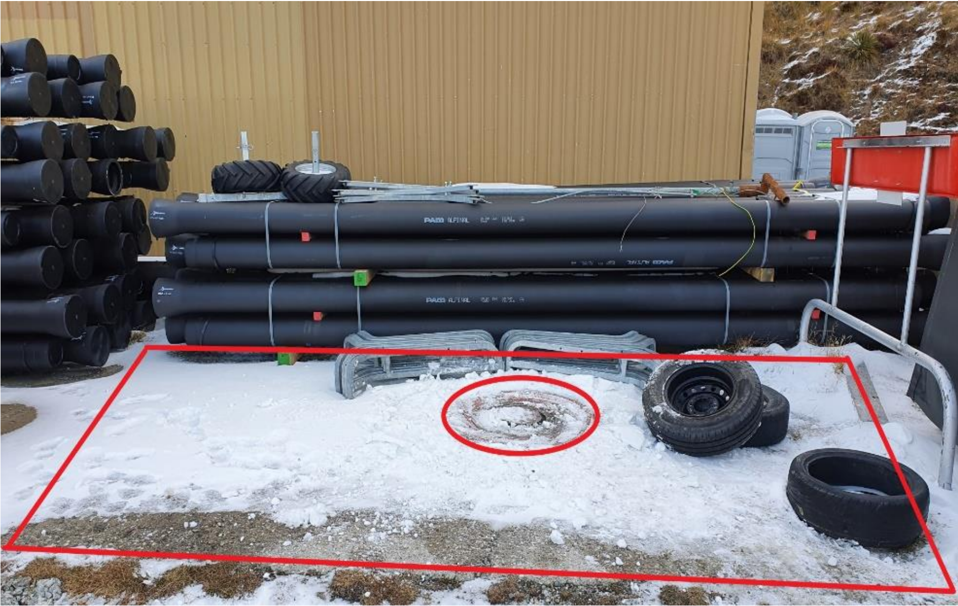
Figure 24 Bulk Fuel Storage - Diesel (in ground tank)
