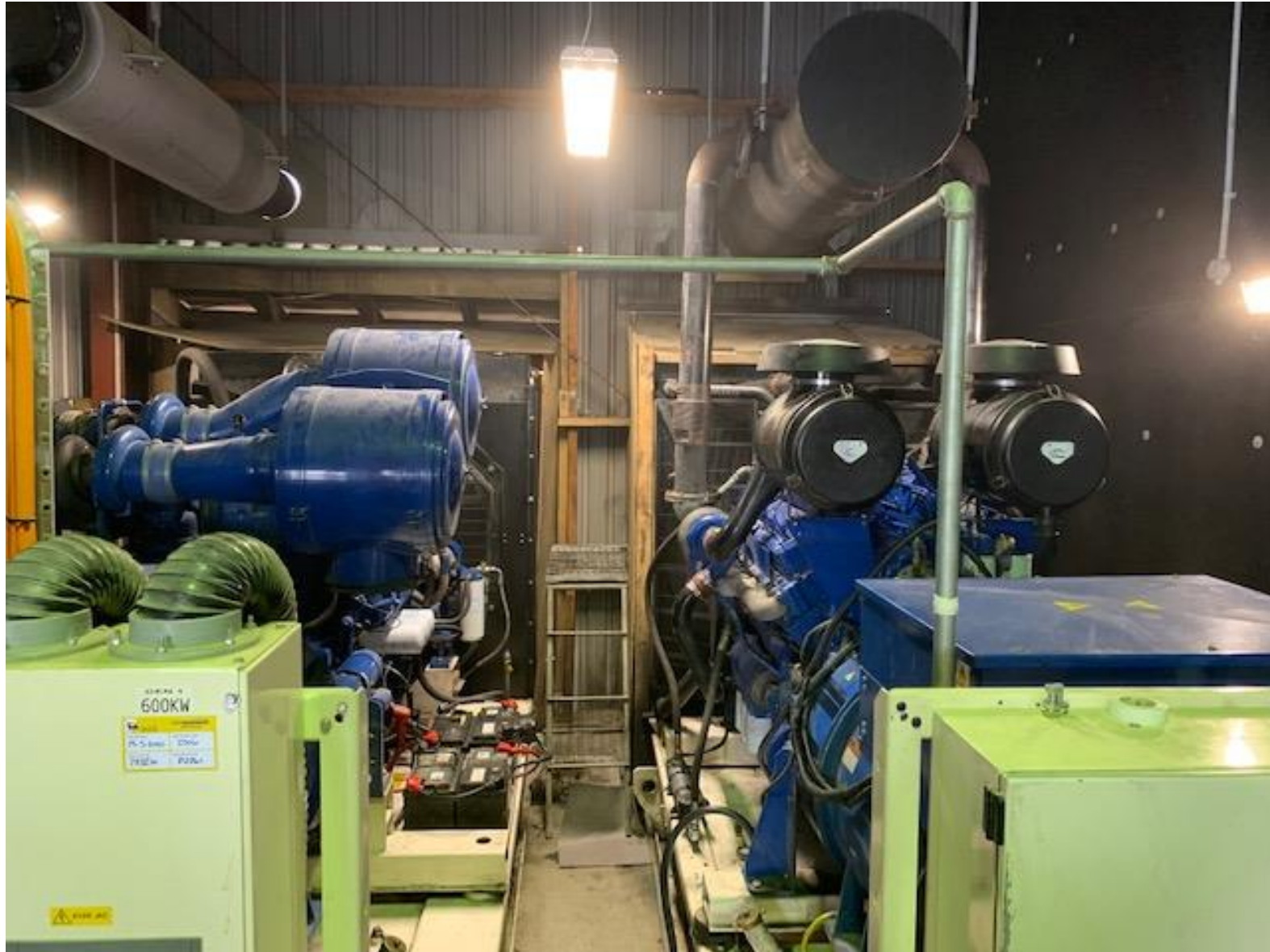
Figure 25 Backup generator (in Snow Groomer Shed)
