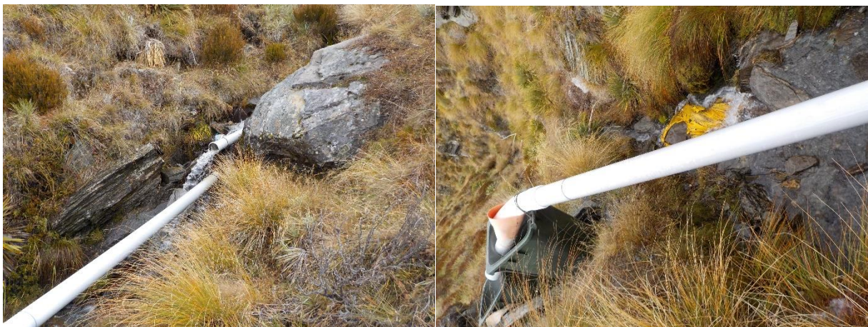
Figure 9: Site CONE10 with the water intake looking upstream (left) and downstream (right).
