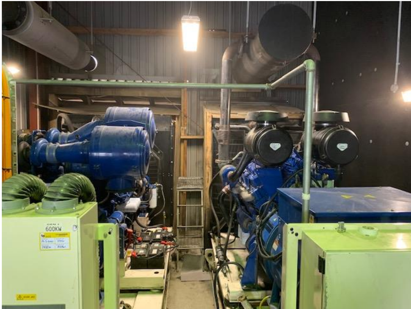
Figure 25 Backup generator (In Snow Groomer Shed)
