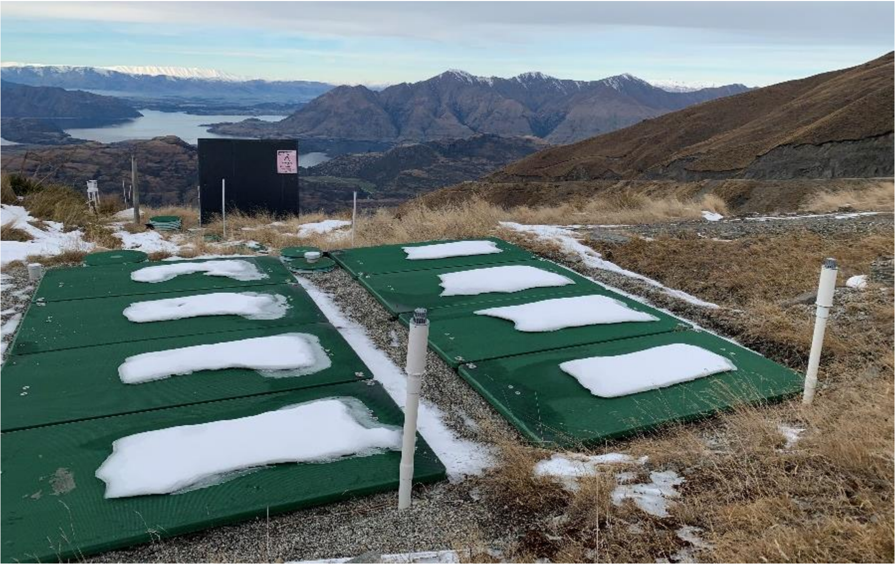
Figure 34 Wastewater Treatment Plant (incl pump shed)
