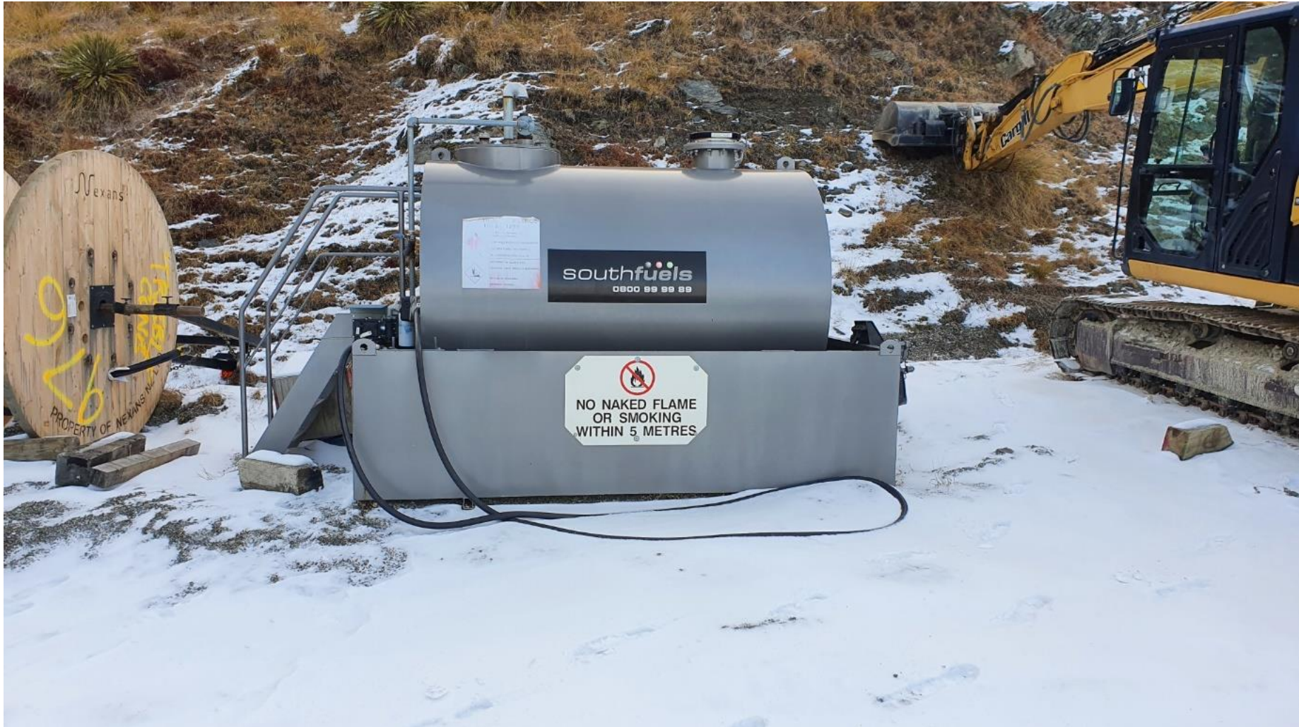
Figure 23 Bulk Fuel Storage – Petrol
