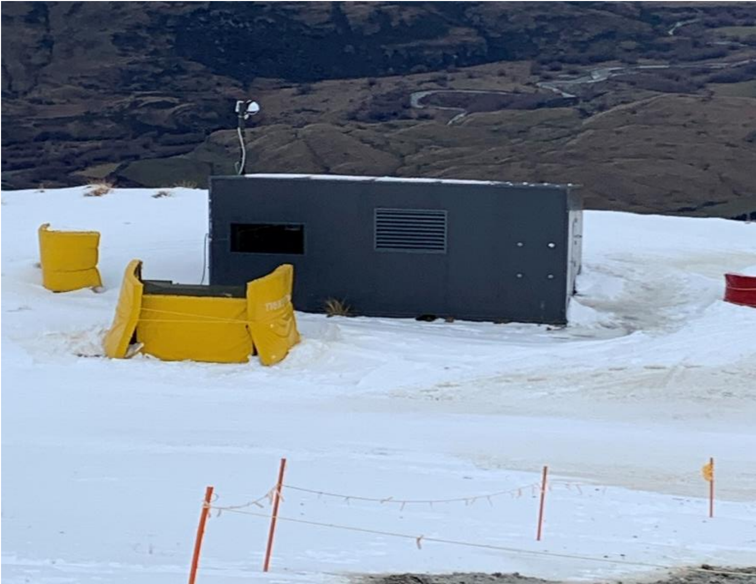
Figure 55 Mid Mountain Booster pump station
