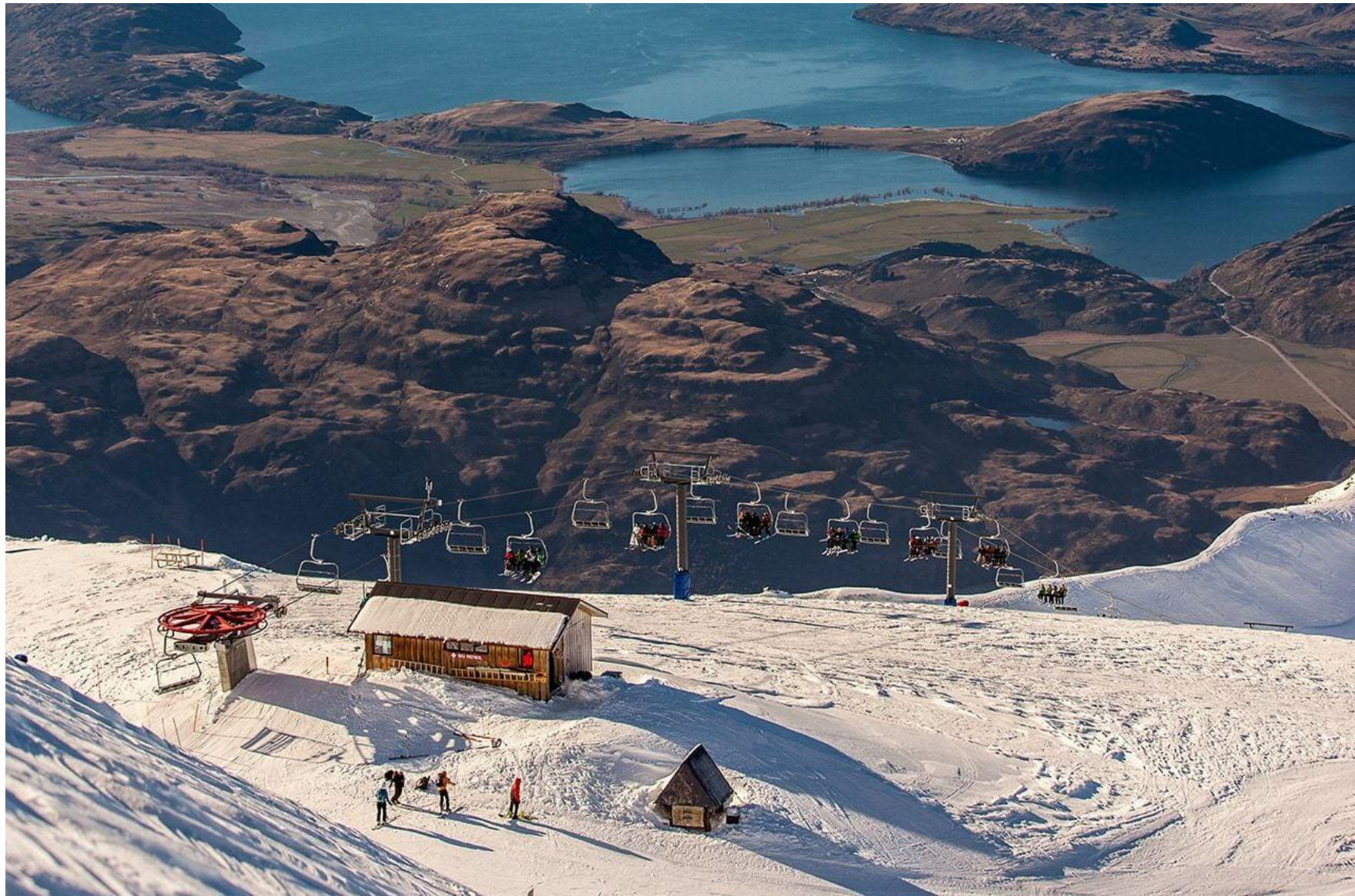
Figure 60 Top of Quad lift – Return station, operator / patrol hut and small 'A' Frame Patrol Equipment Shed
