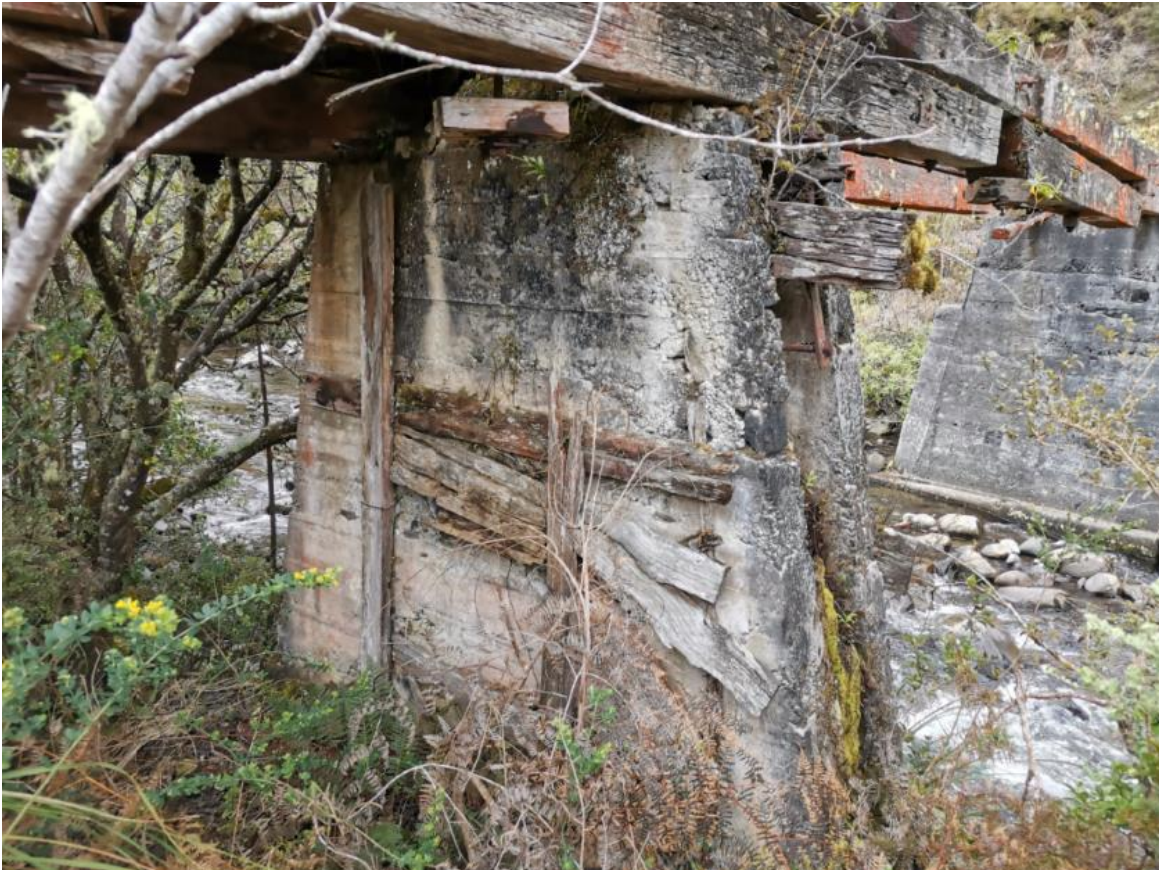
Photo of existing abutment/piers of the 34m bridge over the Mangawhero river.
