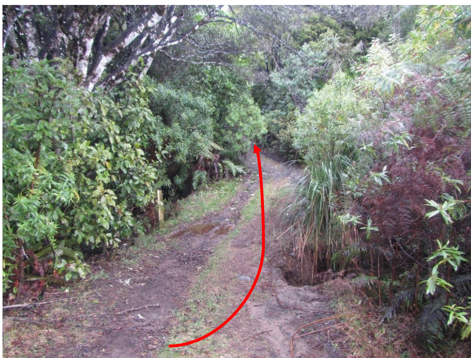
Plate 15: Existing culvert under the gravel road at NZTM E1809687 N5637728. Broadleaved indigenous forest is present on both sides of the gravel road. Red arrow indicates the direction of Ohakune. 16 September 2021.
