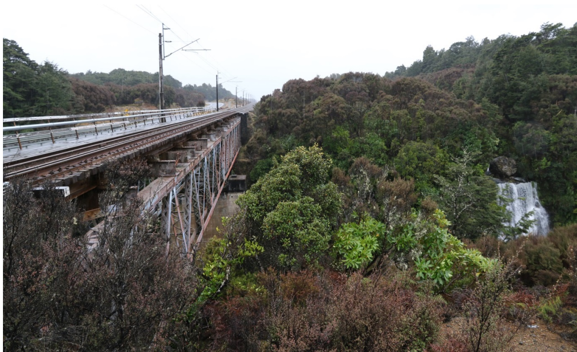
Figure 16 Mangaturuturu rail viaduct and road (left) viewing across gorge to attractive waterfall opposite.
