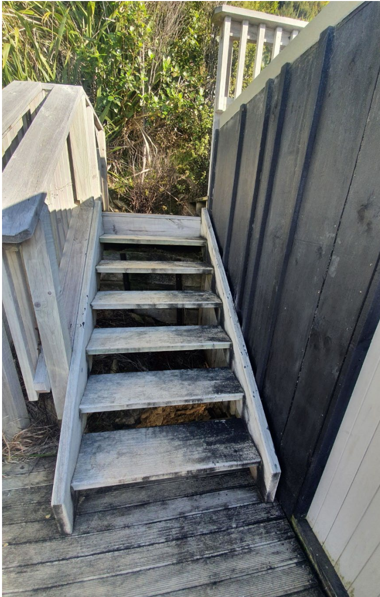
Photos of the structures under the application for McKendry, Paul Francis; King, Gregory John and McKendry, Matthew Leo
