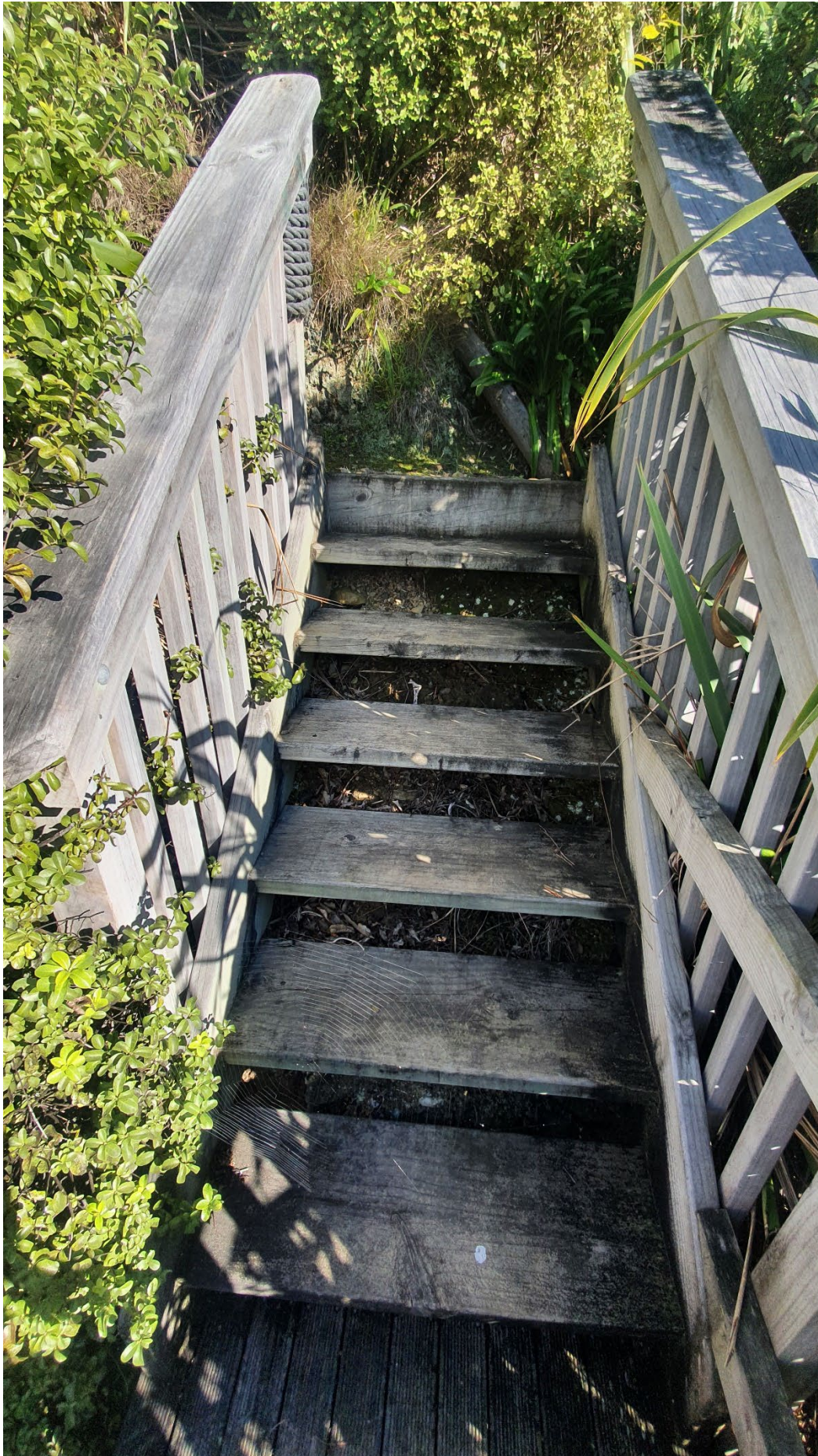
Photos of the structures under the application for McKendry, Paul Francis; King, Gregory John and McKendry, Matthew Leo
